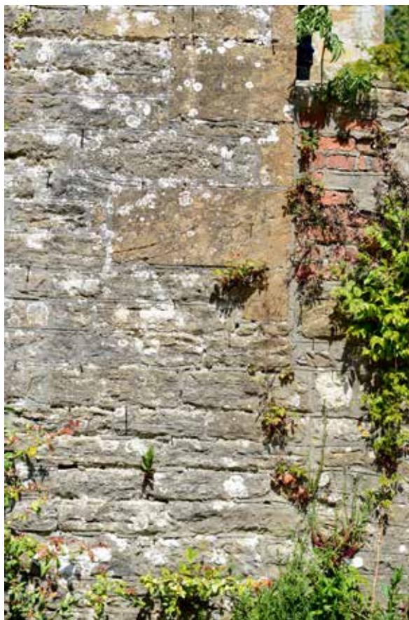
7. Detail of the masonry from the east end of the south front of the main block.
