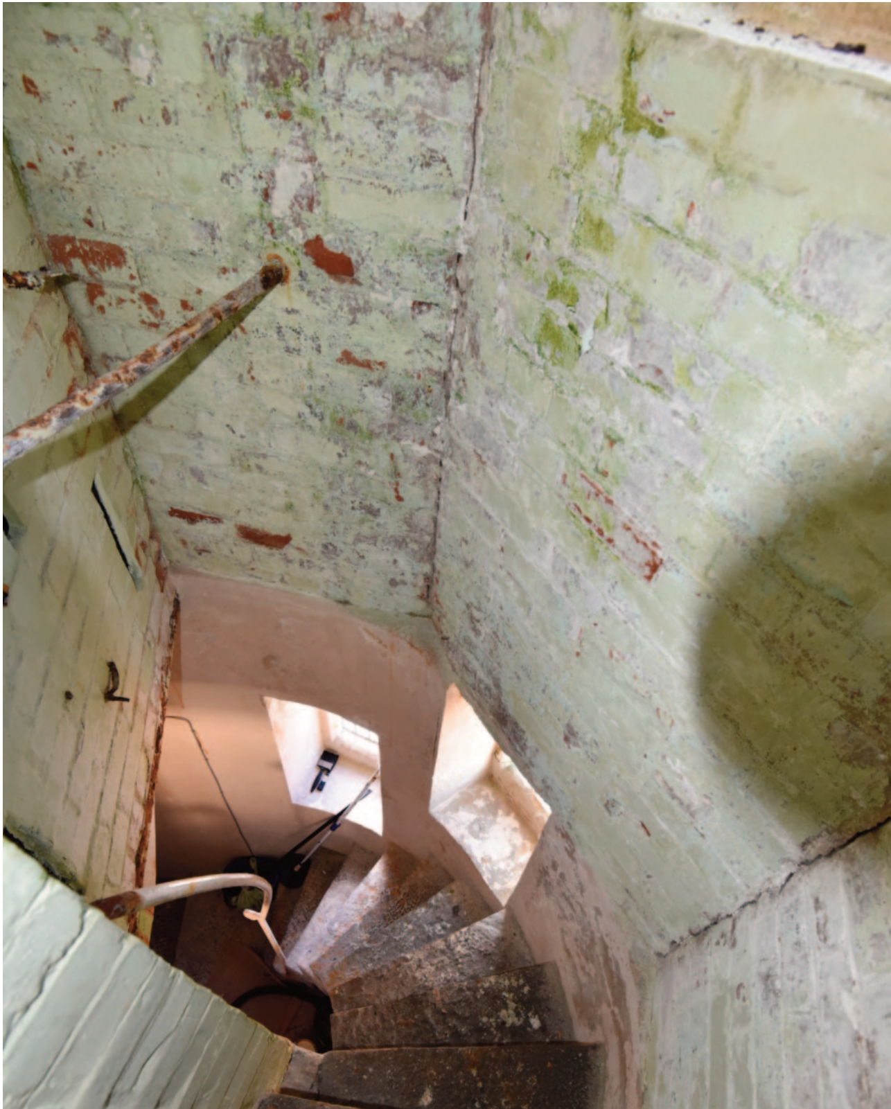
Fig. 27. The tower stairs seen from the upper room. The inner face of the walls are lined with brick with steel reinforcing to the stair opening and the tower roof.
