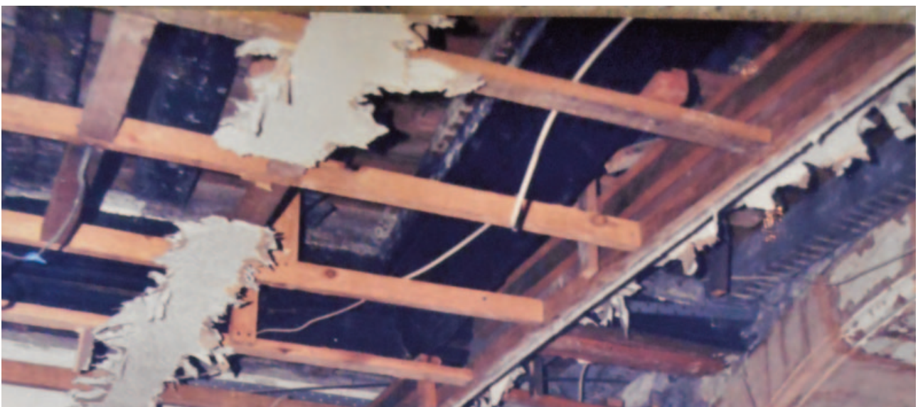
Fig. 22. A second view shows the ceiling beam attached to a cross beam both of which are in-situ but cut back when the building was refronted and narrowed by Vials. In situ floor joists can be seen on the left.
