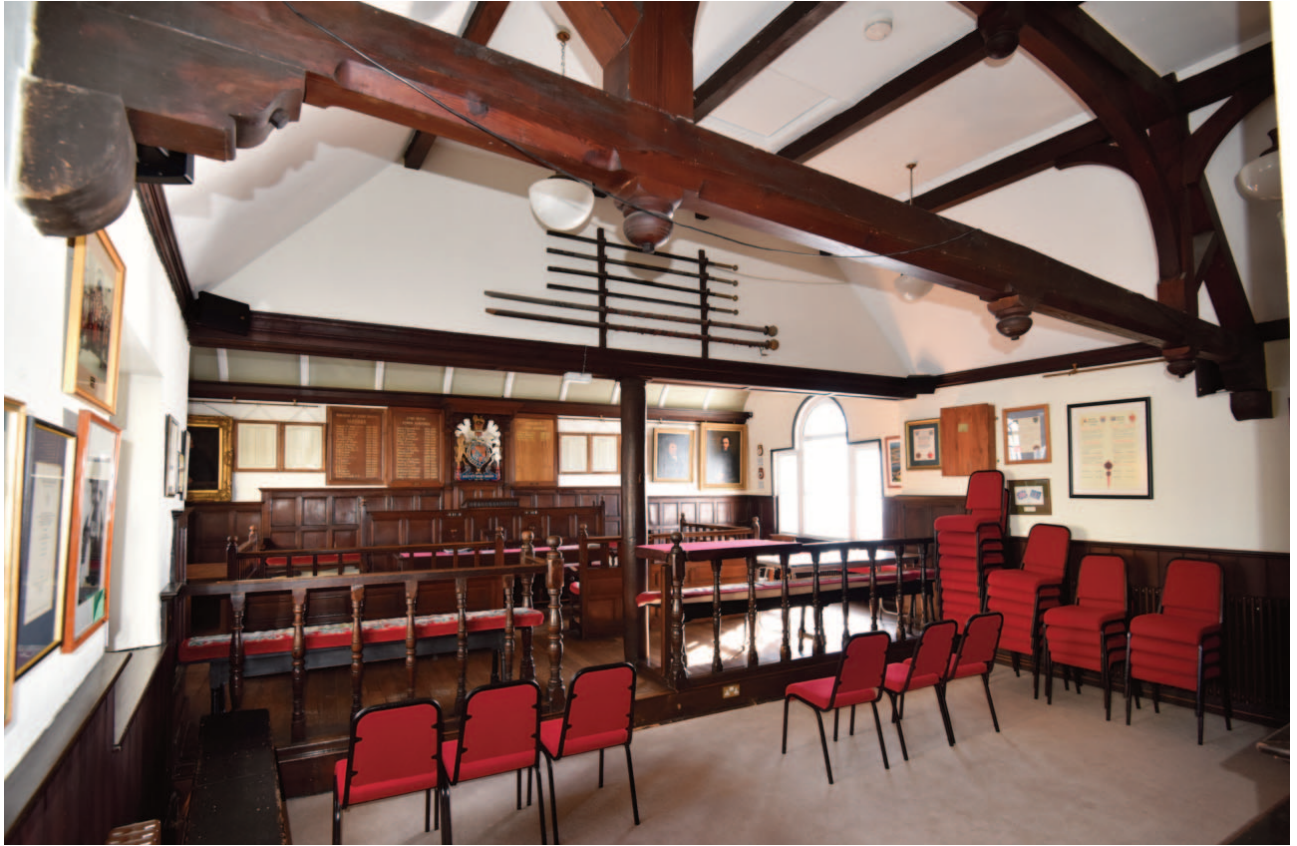
Fig. 26. The first floor meeting room, with the late 19th century truss in the foreground. The circular post supporting the downstand is historic; and the structure beyond this forms part of the earlier building. .
