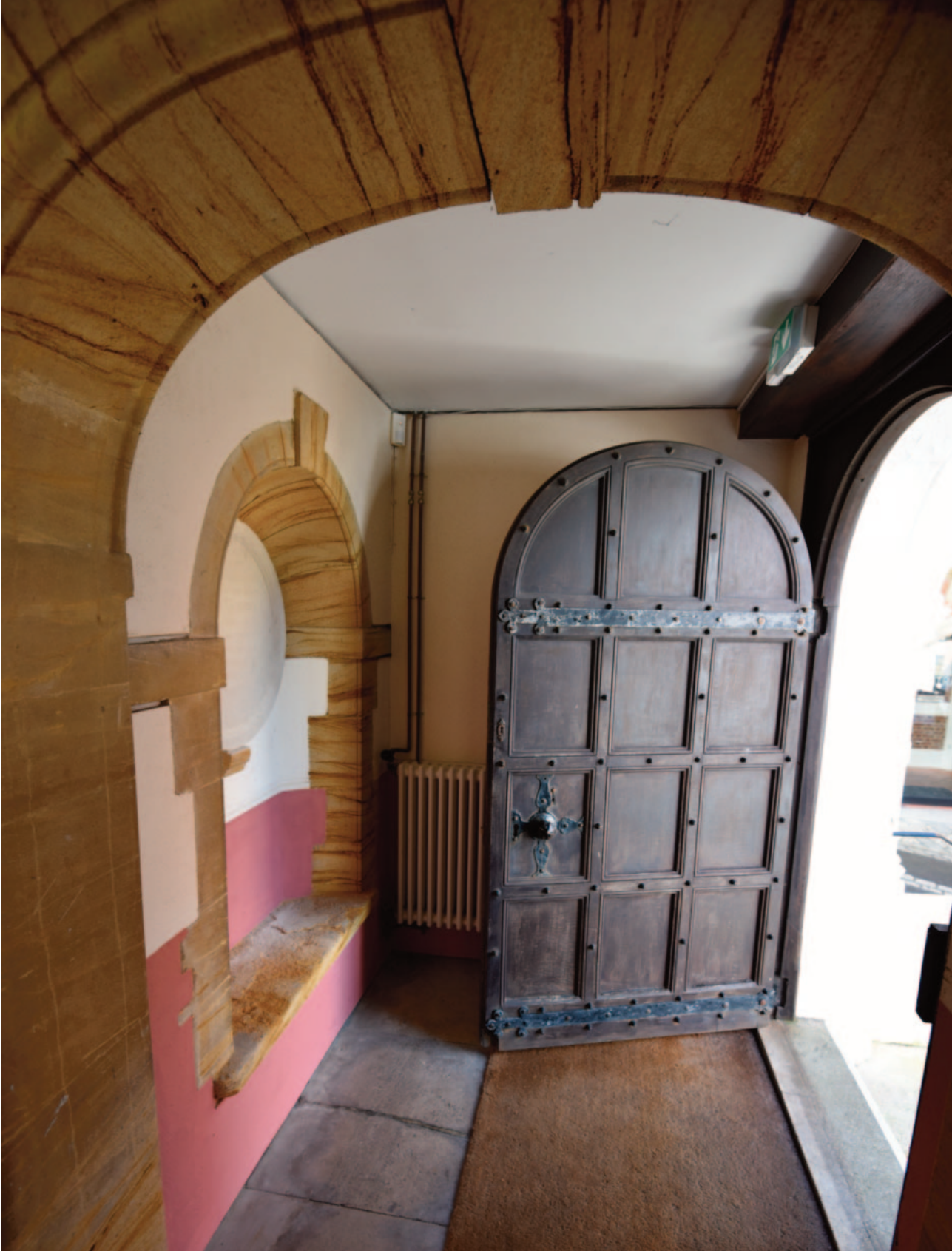
Fig. 24. The good quality Victorian entrance door opens into the small entrance lobby with its decorative stone detailing and commemorative plaque within the arched alcove.
