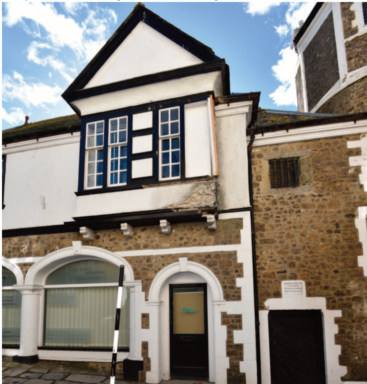
Fig 14. The oriel window showing recent vehicular impact damage. The rendered panels and much of the lower framework is of modern construction following repeated vehicle damage.
