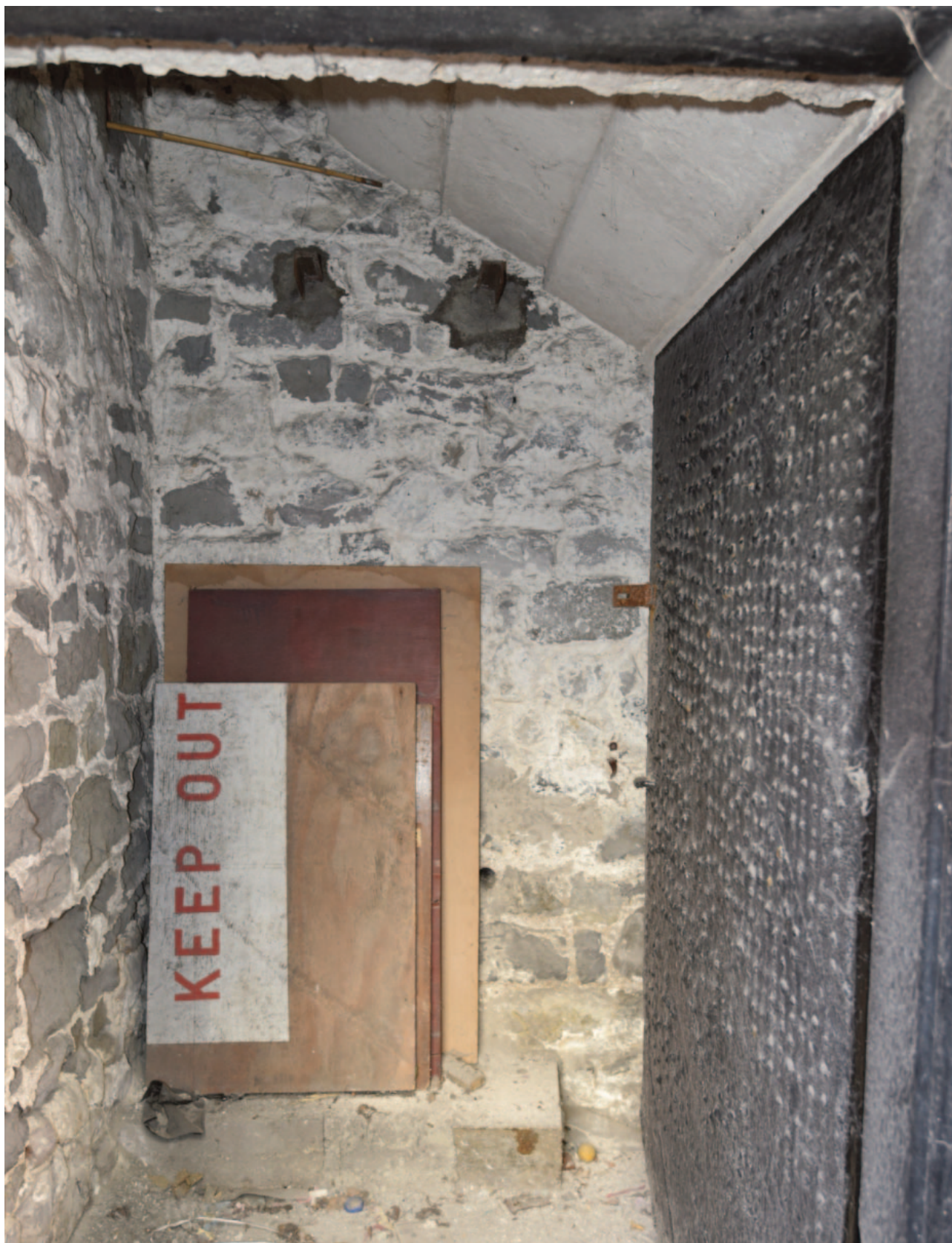
Fig. 23. The remnant of the former town gaol survives in truncated form with the historic entrance door reset in the repositioned front wall. The stairs to the Council chamber cut through its original roof.
