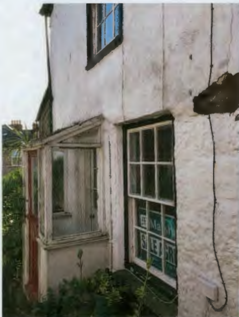
Front of property showing dilapidated porch.
