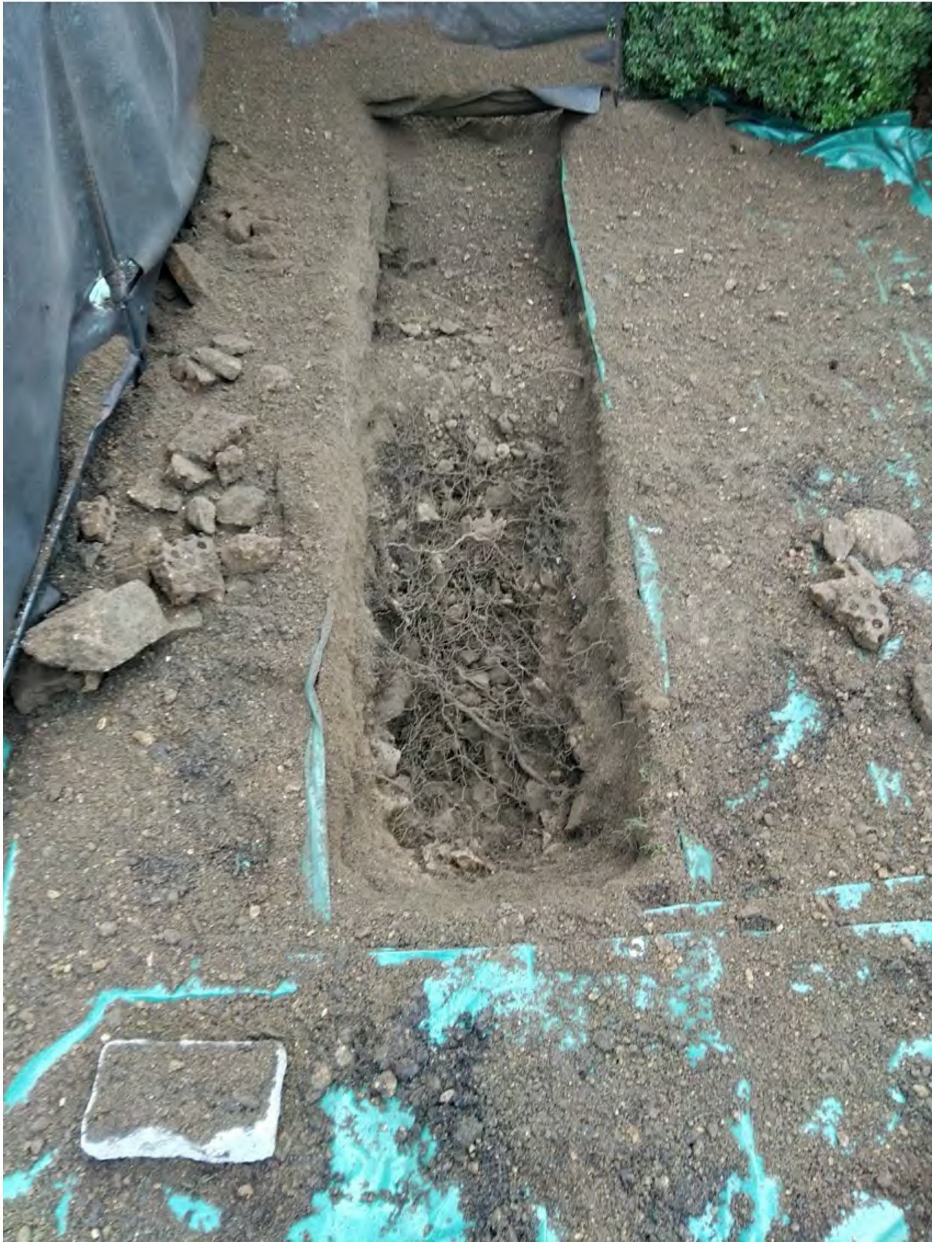
Image 5: Showing 'Section 4' of the trench open with the brick rubble removed and a dense area of fibrous root growth.
