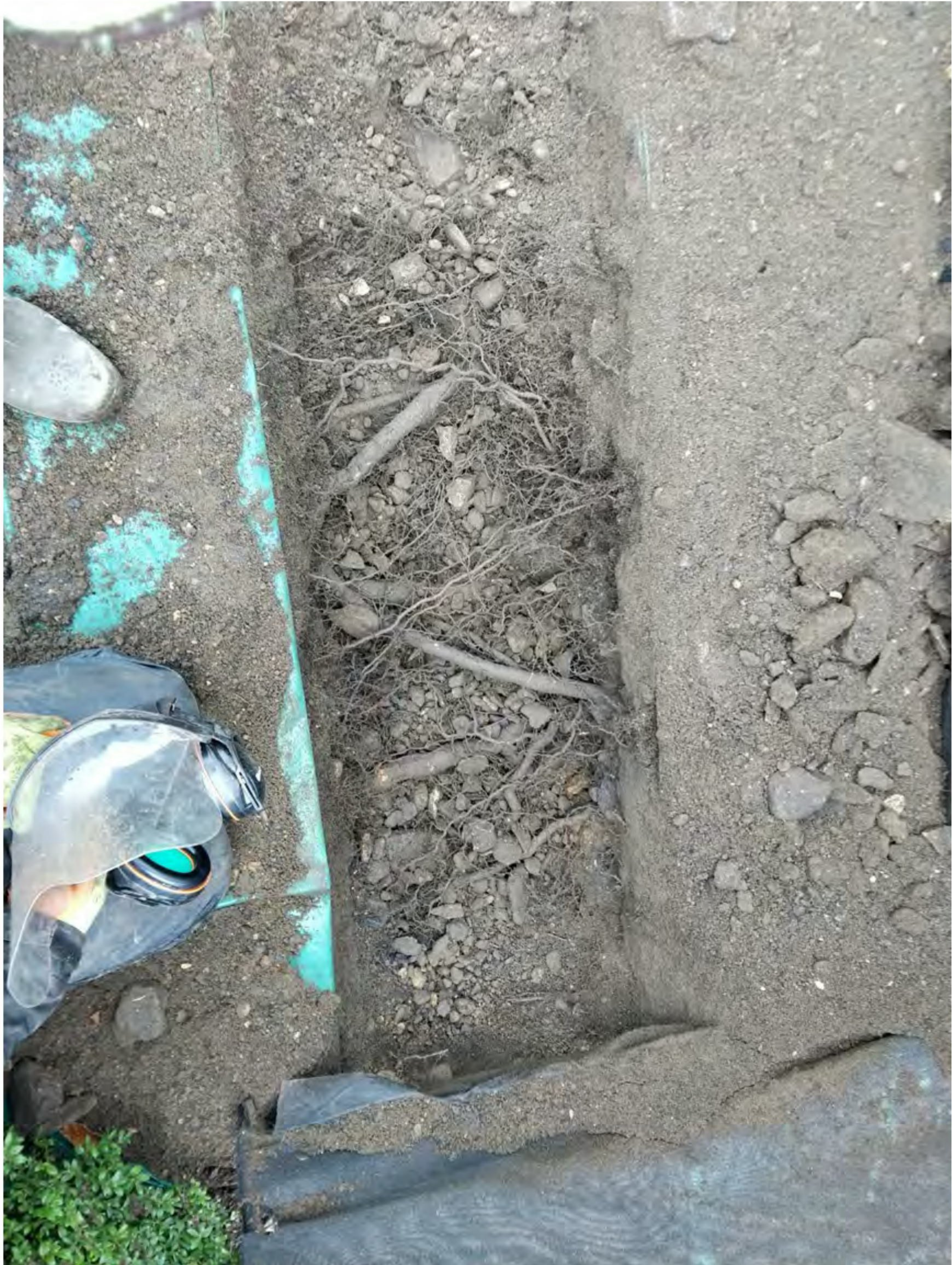
Image 4: Showing 'Section 4' of the trench open with the brick rubble removed and 6No. roots at 200-300mm down. Each of these in the range 10-40mm diameter.
