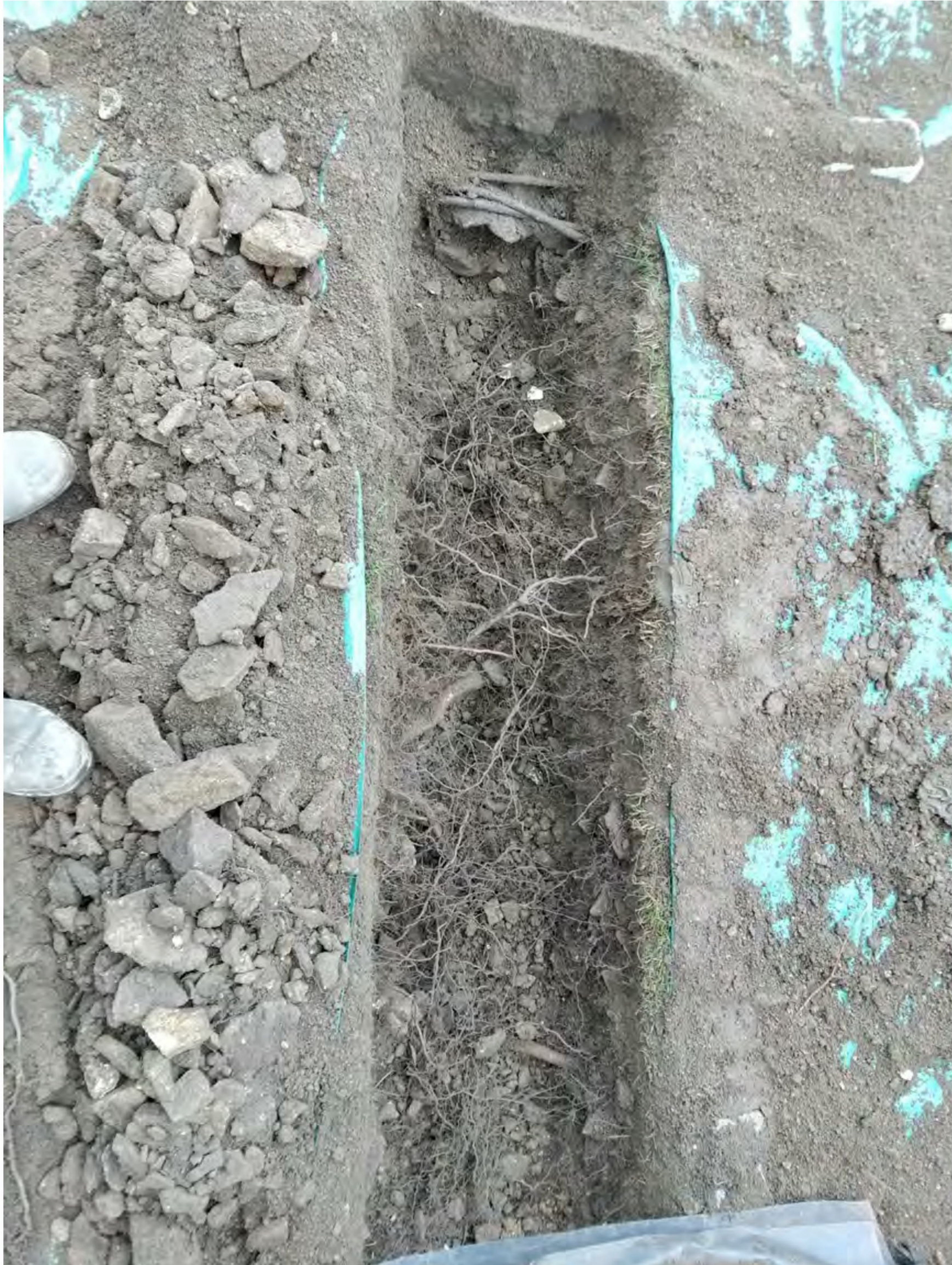
Image 2: Showing 'Section 1' of trench open. The retaining wall to the wider lawn area is located out of sight but at the top of the frame.
