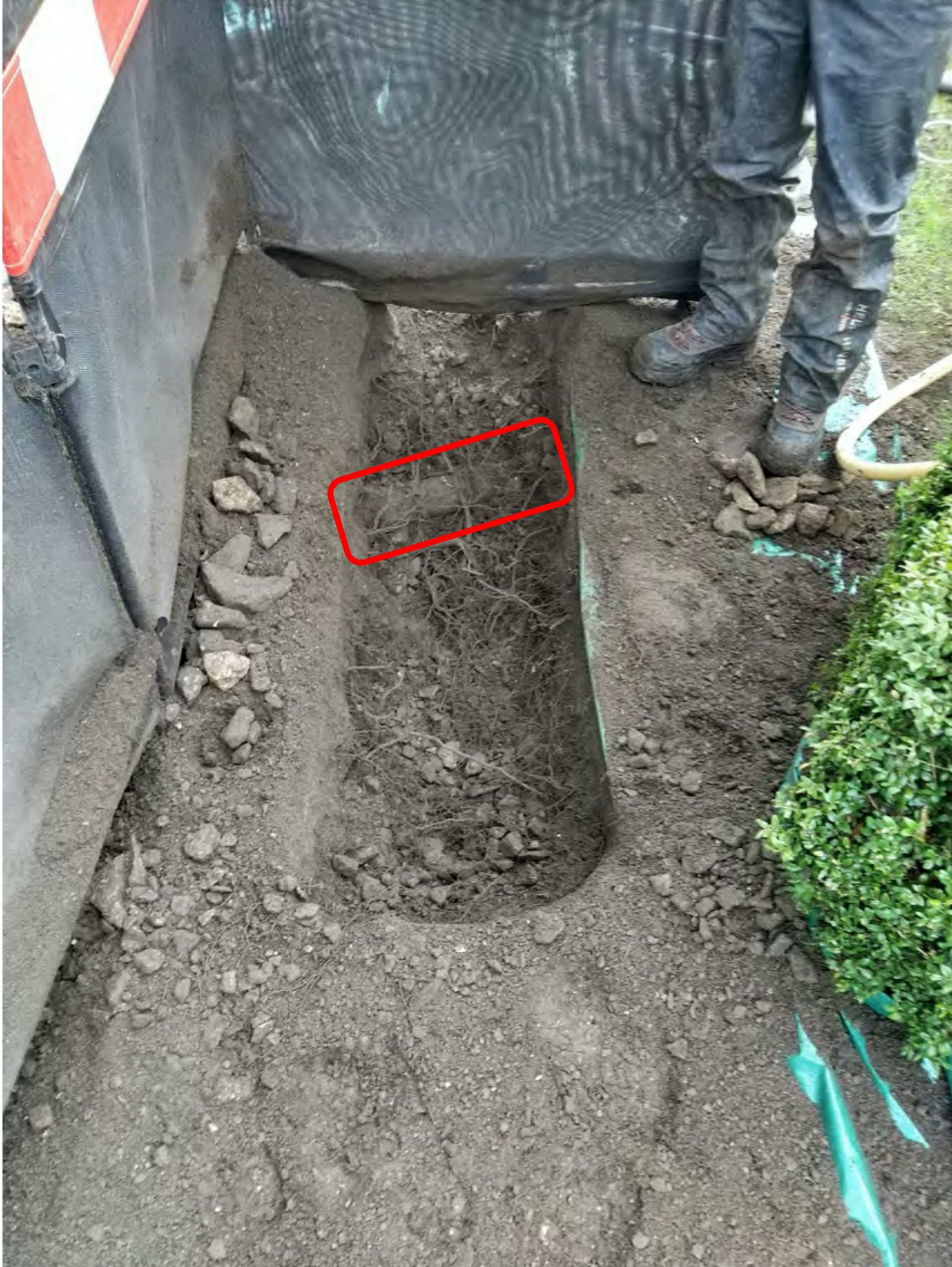
Image 3: Showing 'Section 2' of the trench open. The first significant root was encountered in this section of trench - as highlighted by the red rectangle.
