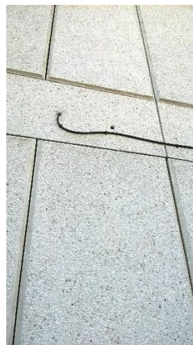
Figure 3: Hole on east elevation
