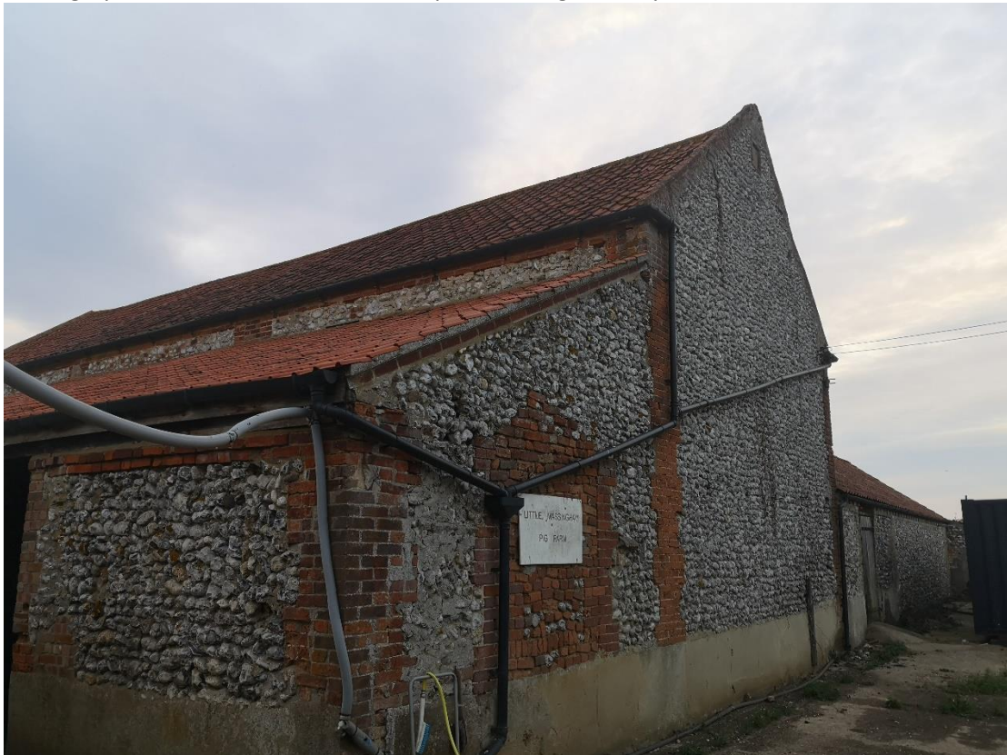
Photograph 4: Eastern aspect of the barn look north from the south eastern corner – edge of metal container cabin
