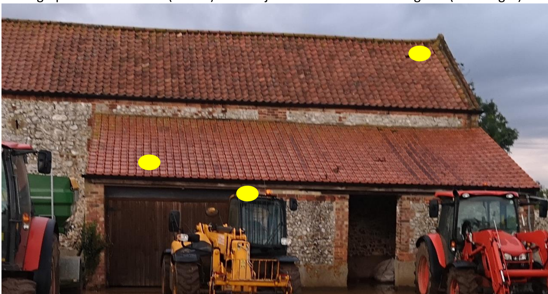
Photograph 6: Zoomed photo (photo 1) of roof to highlight emergence locations depicted by yellow circles
