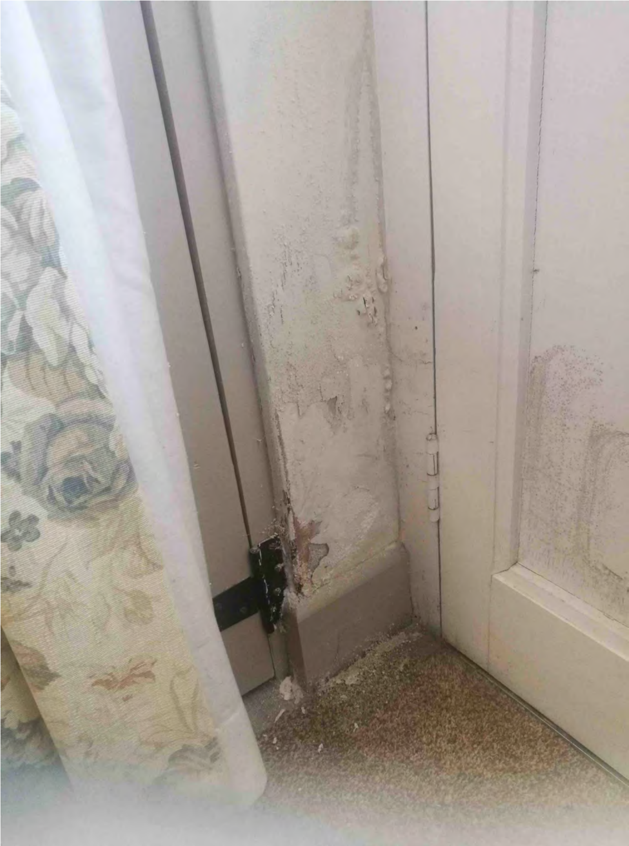
Photo of ground floor southern external door; water ingress damage to plasterwork.
