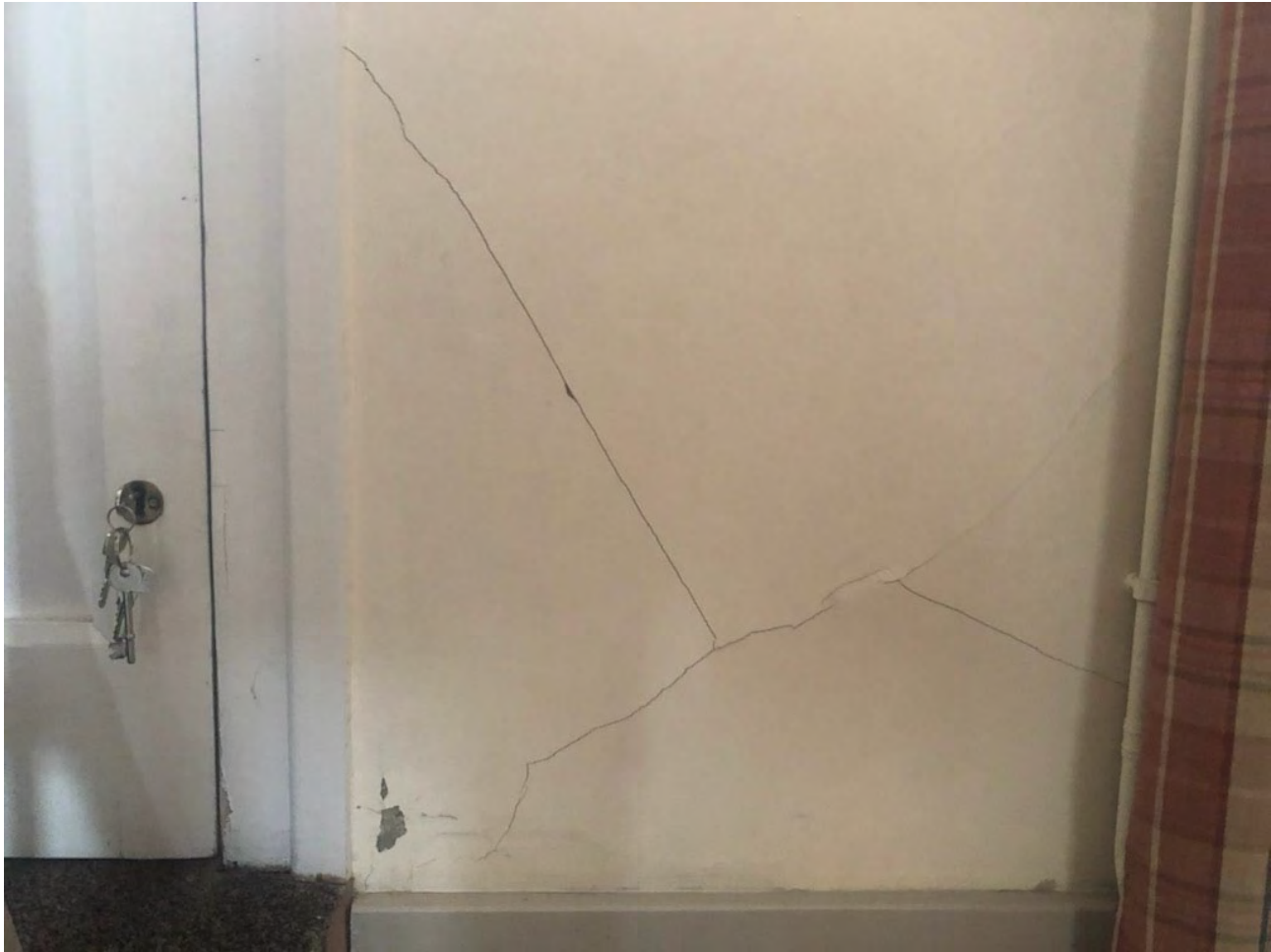
Photo of ground floor northern external door; water ingress damage to plasterwork, heavily cracked.
