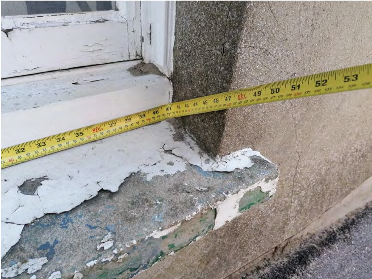
Photo of ground floor window cill; deteriorating window and frame along with cracked adjacent render.
