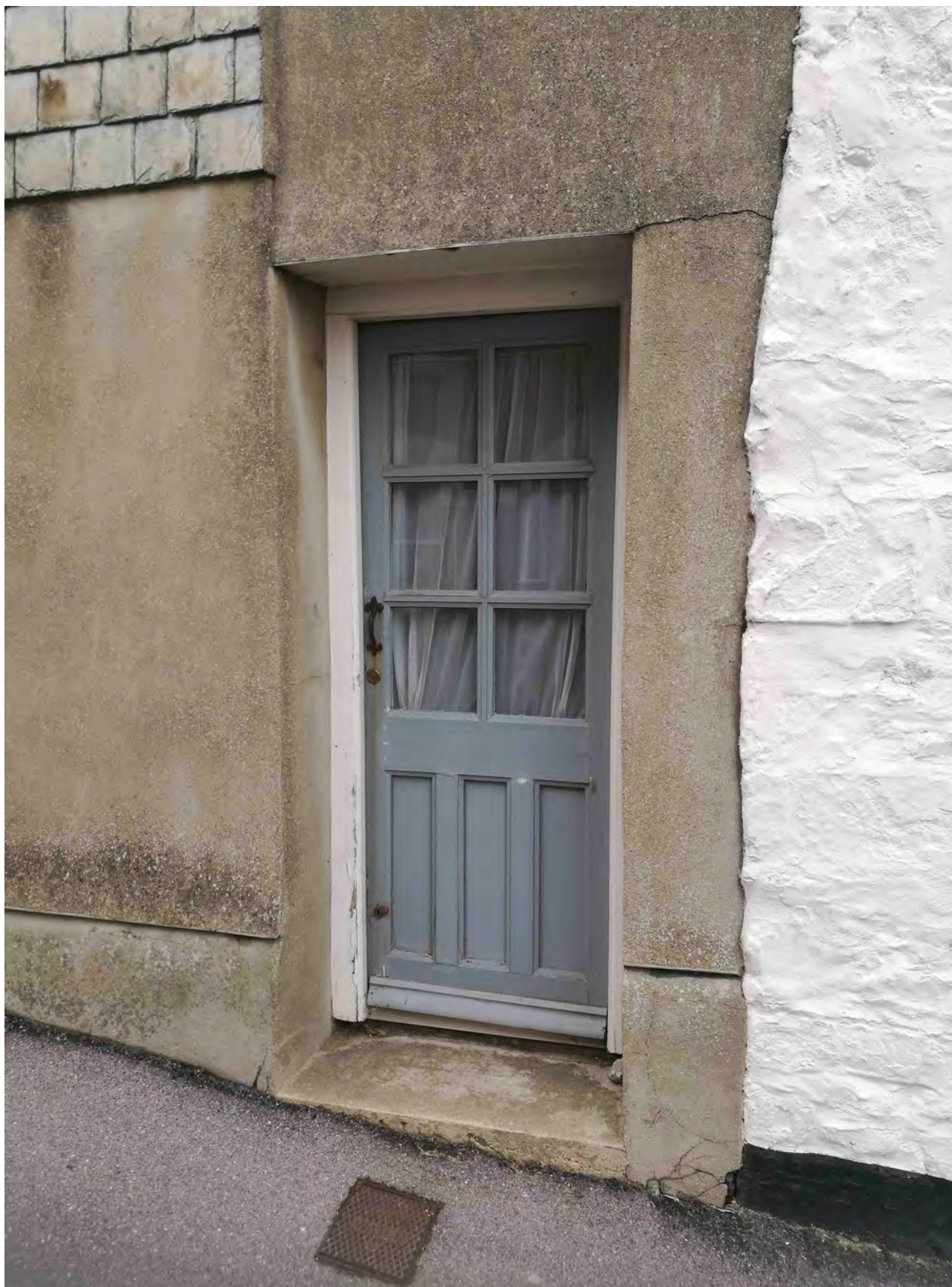
Photo of southern external door; deteriorating door and frame along with cracked adjacent render.
