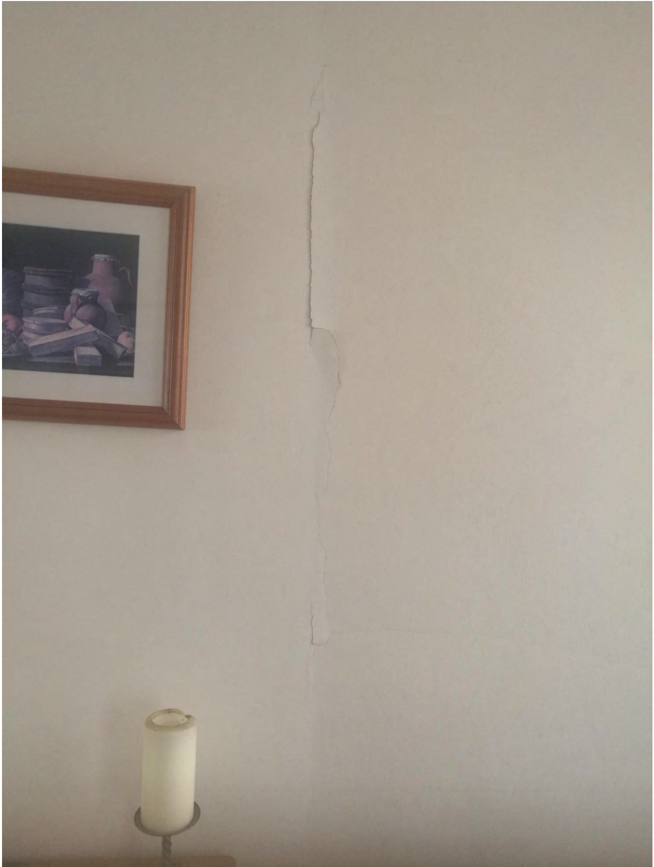
Photo of internal dining room wall with cracked plasterwork.
