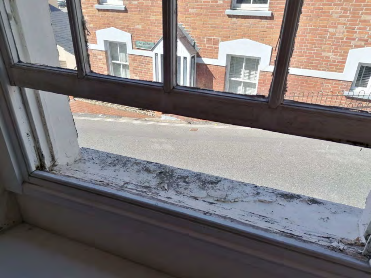
Photo of first floor bedroom window; deteriorating window, cill and frame.
