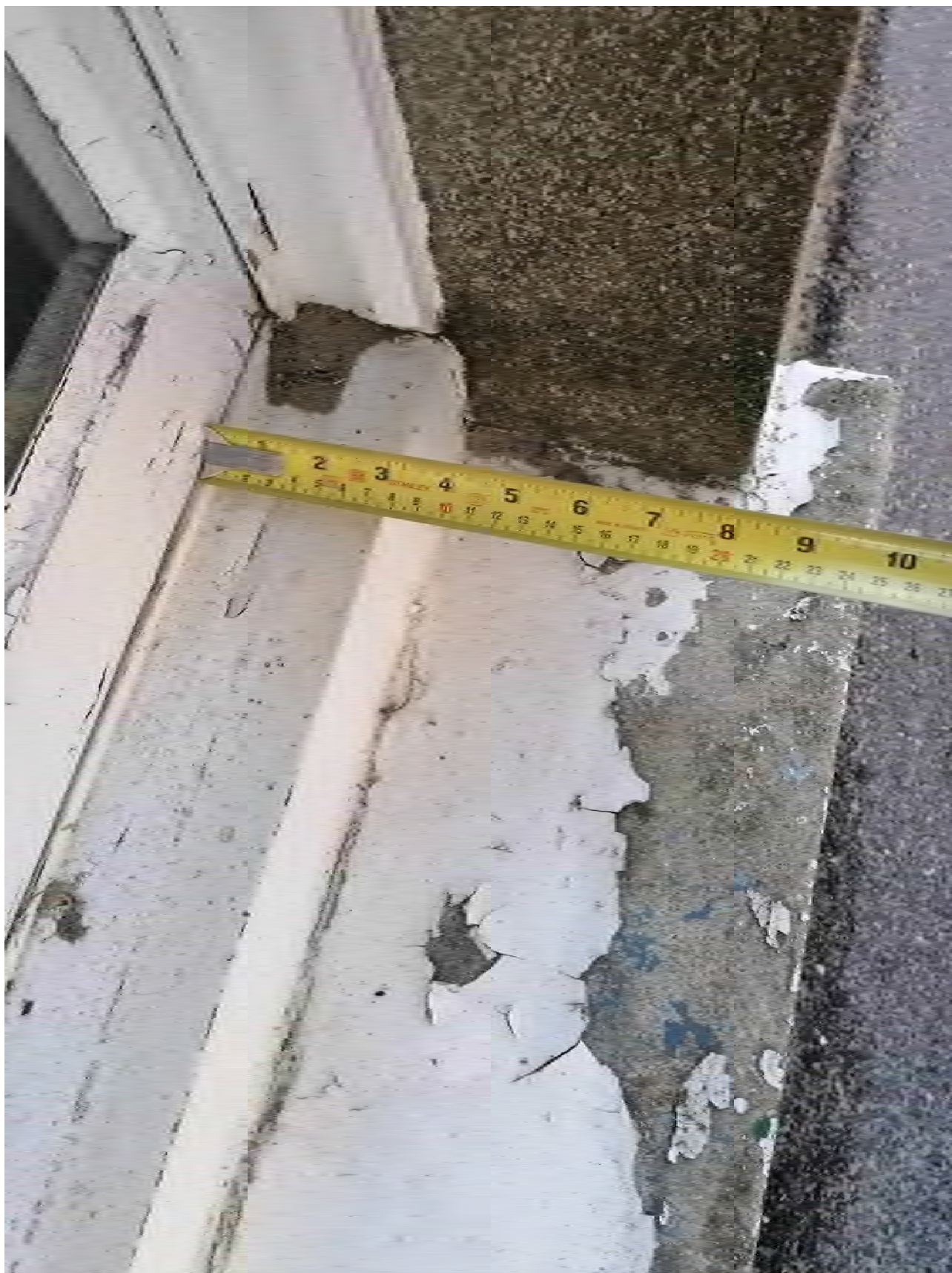
Photo of ground floor window cill; deteriorating window and frame along with cracked adjacent render.
