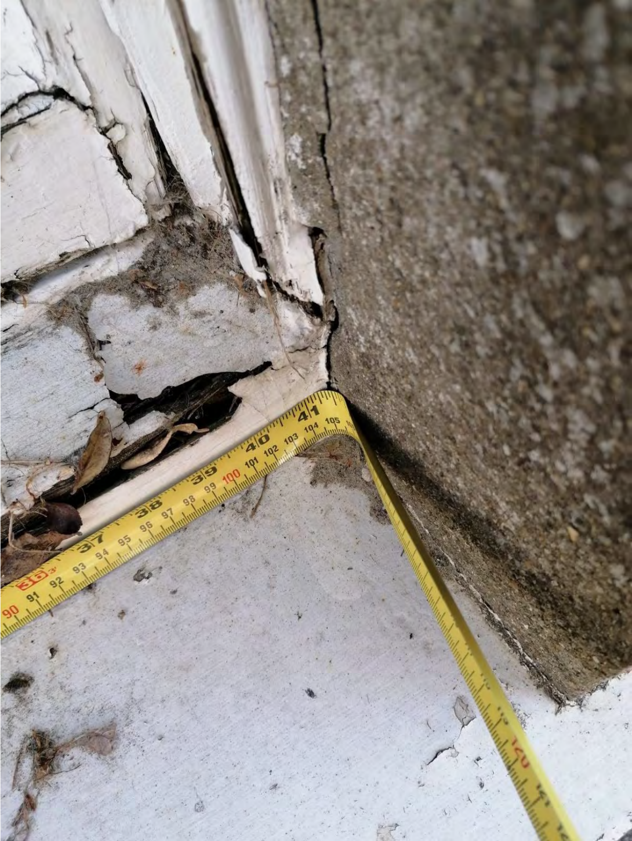
Photo of first floor bedroom window cill; deteriorating window and frame along with cracked adjacent render.
