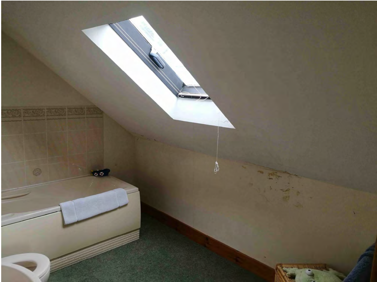
Photo of first floor bathroom rooflight; cracked plasterwork along with water damage to external wall.
