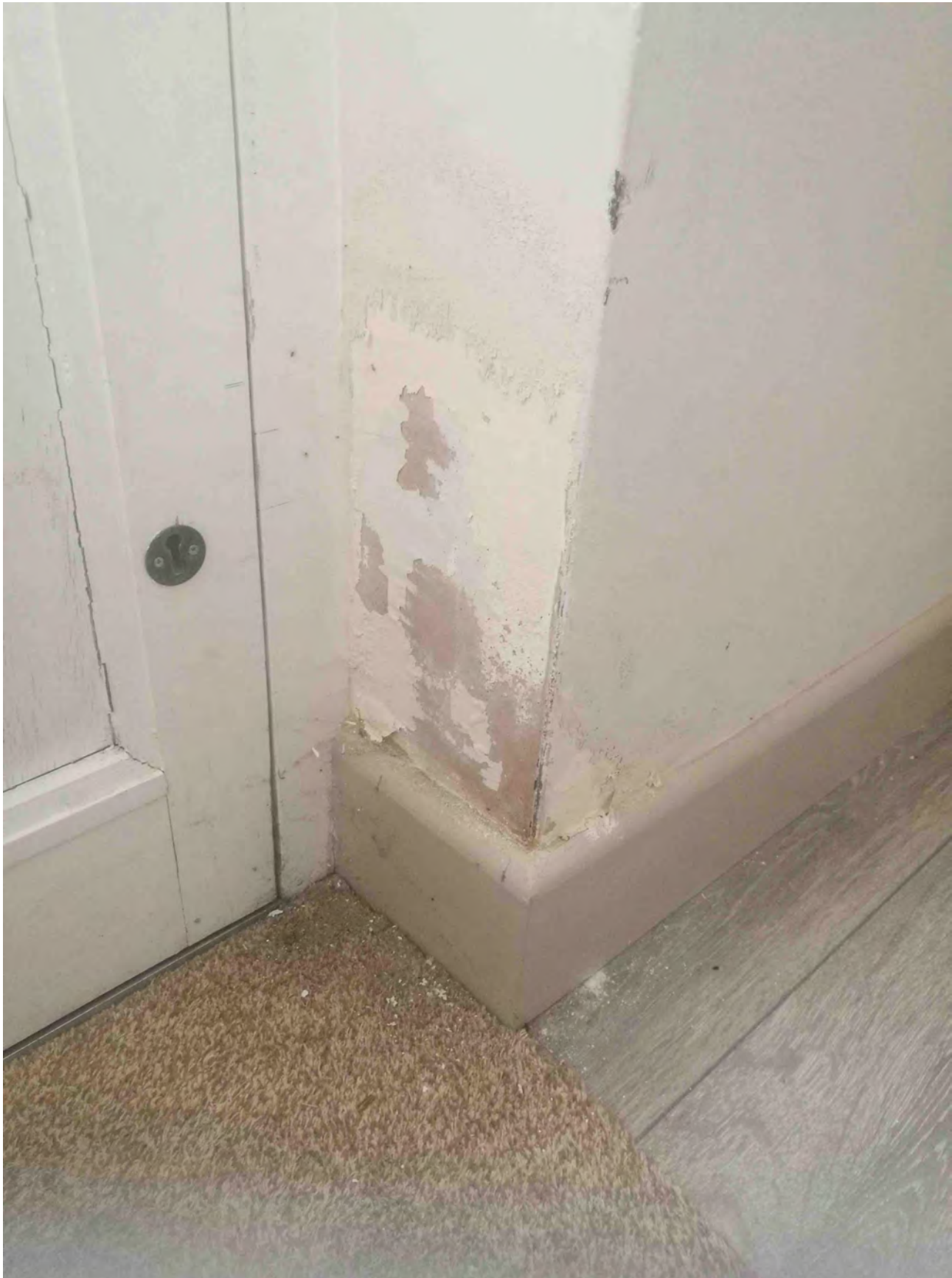
Photo of ground floor southern external door; water ingress damage to plasterwork.
