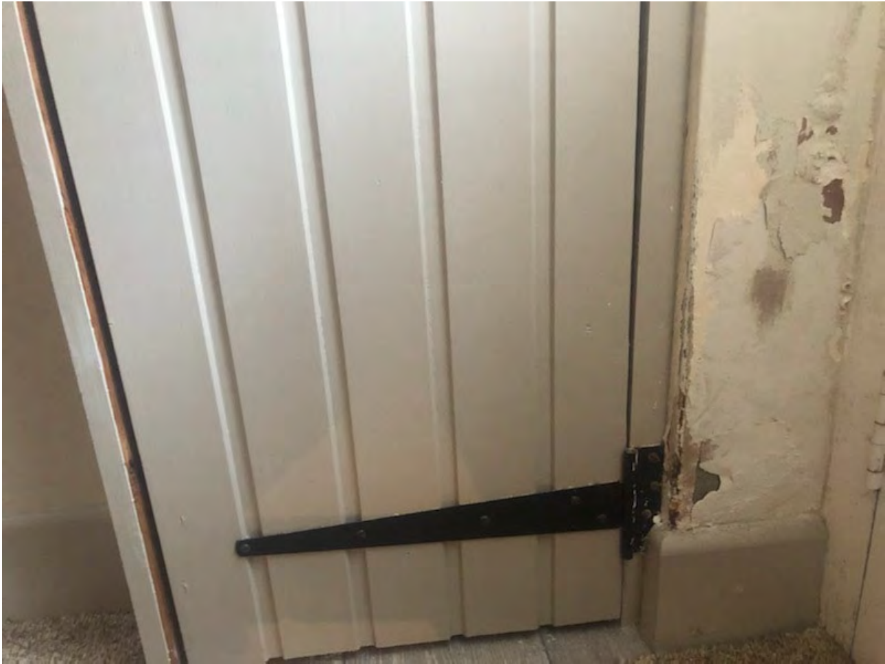
Photo of ground floor southern external door; water ingress damage to plasterwork.
