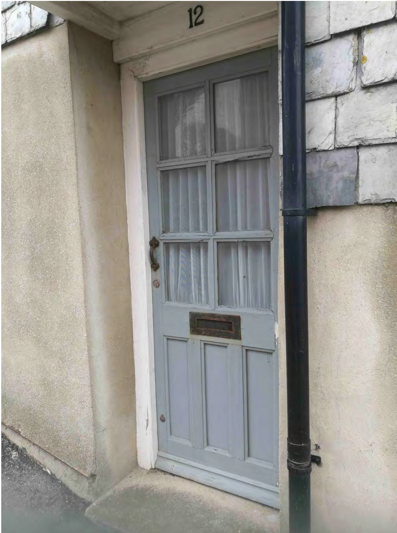
Photo of northern external door; deteriorating door and frame along with cracked adjacent render.
