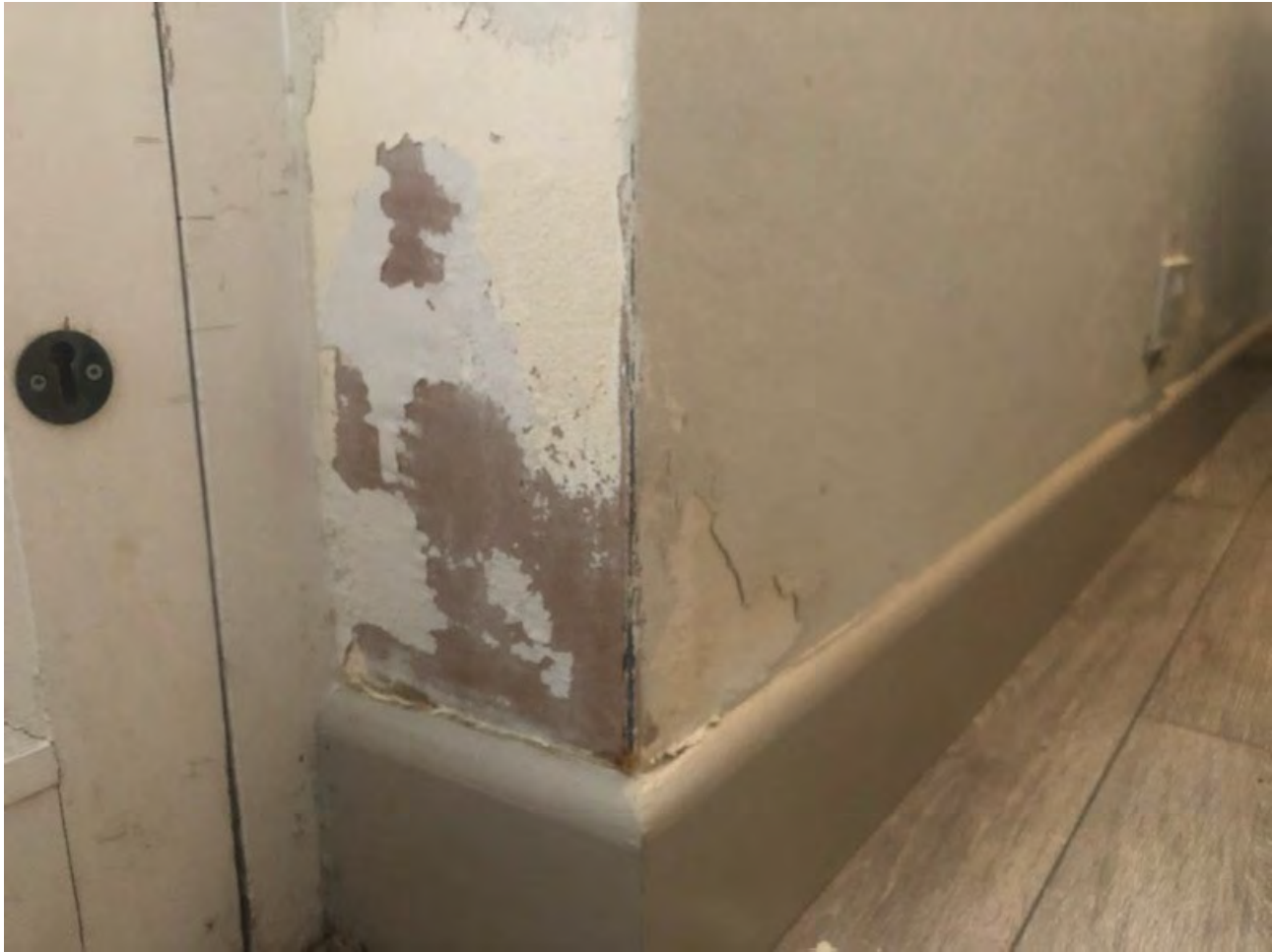
Photo of ground floor southern external door; water ingress damage to plasterwork.
