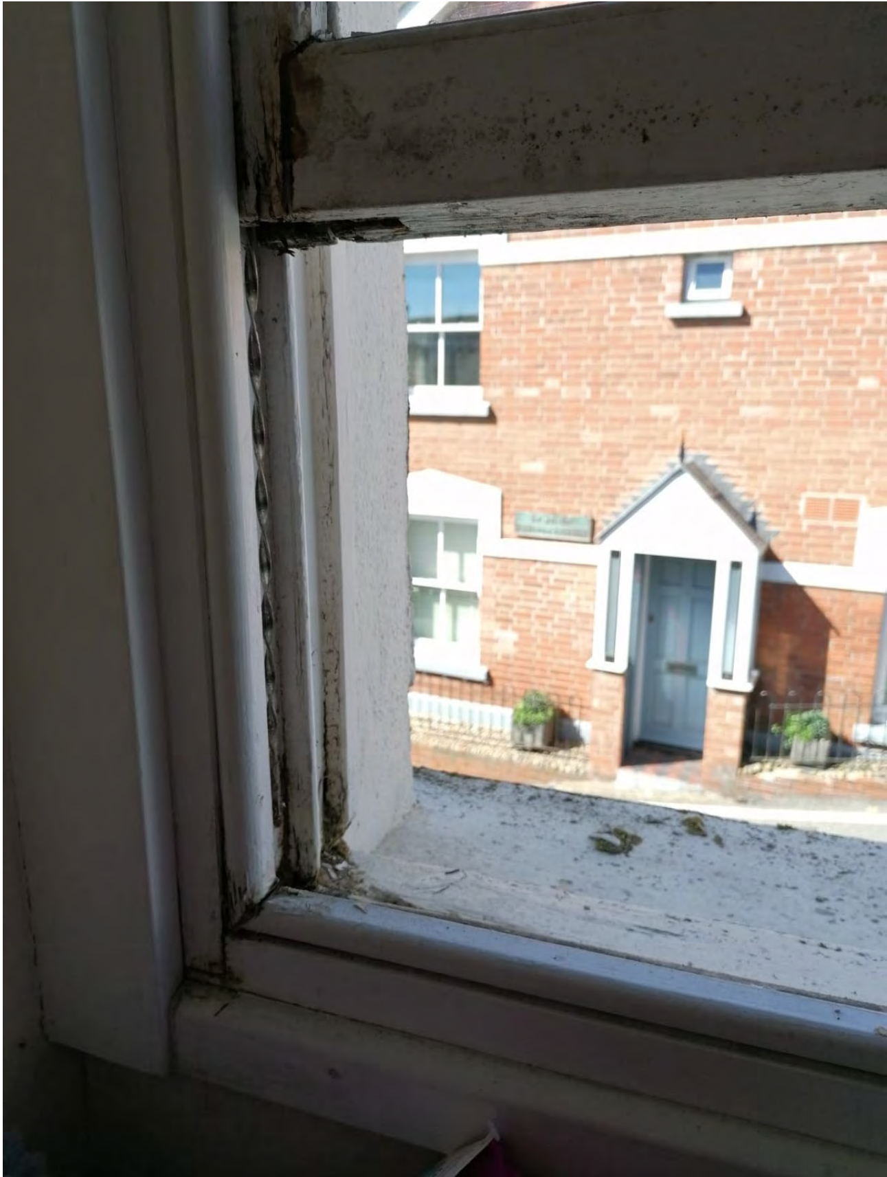
Photo of first floor bedroom window; deteriorating window, cill and frame.
