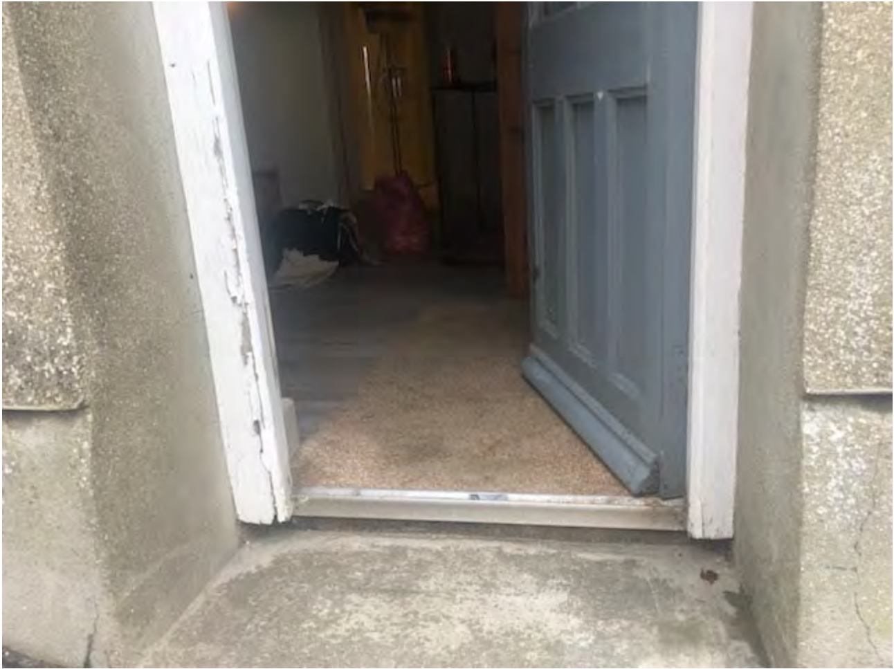
Photo of southern external door; deteriorating door and frame along with cracked adjacent render.
