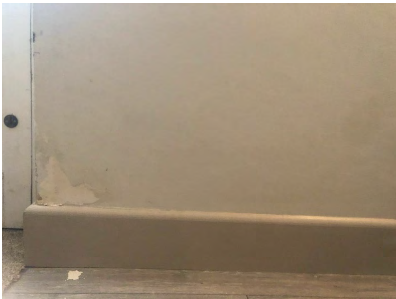
Photo of ground floor southern external door; water ingress damage to plasterwork.
