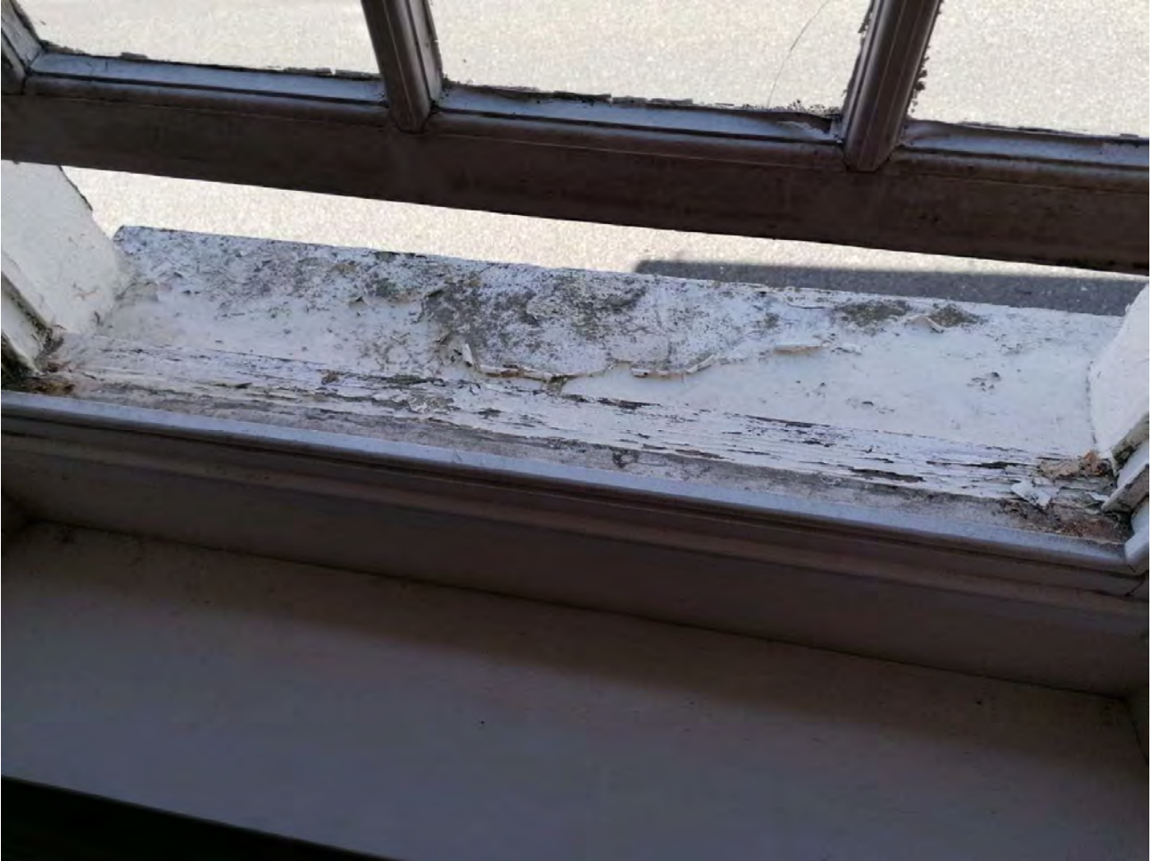
Photo of ground floor window cill; deteriorating window and frame, along with flaking paintwork.
