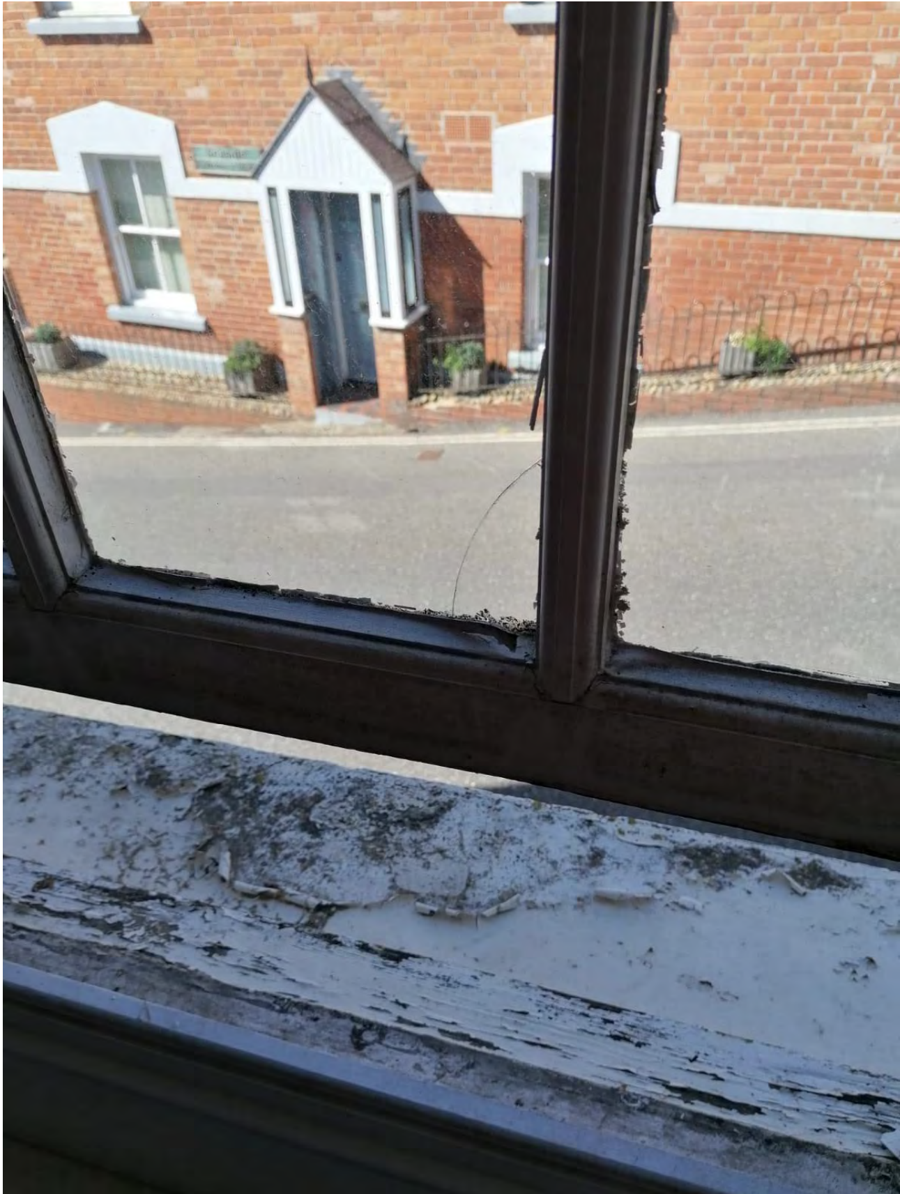
Photo of first floor bedroom window; deteriorating window, cill and frame, along with a cracked pane of glass.
