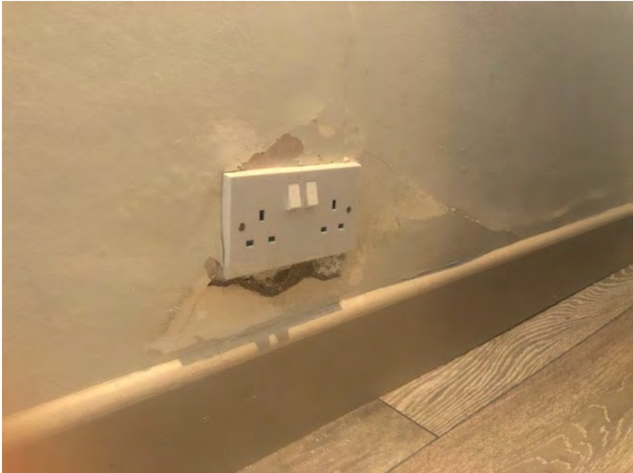
Photo of ground floor external wall; water ingress damage to plasterwork and electrics.
