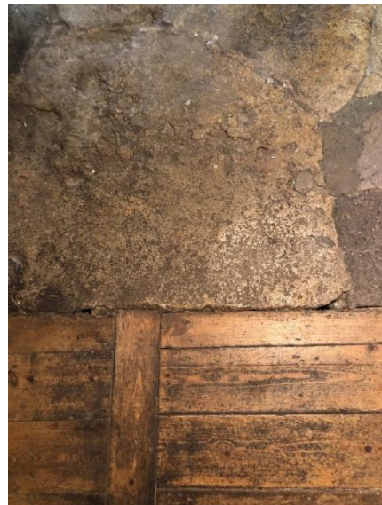
Fig. 2 Close up of the transition between the concrete and timber floor finishes.
