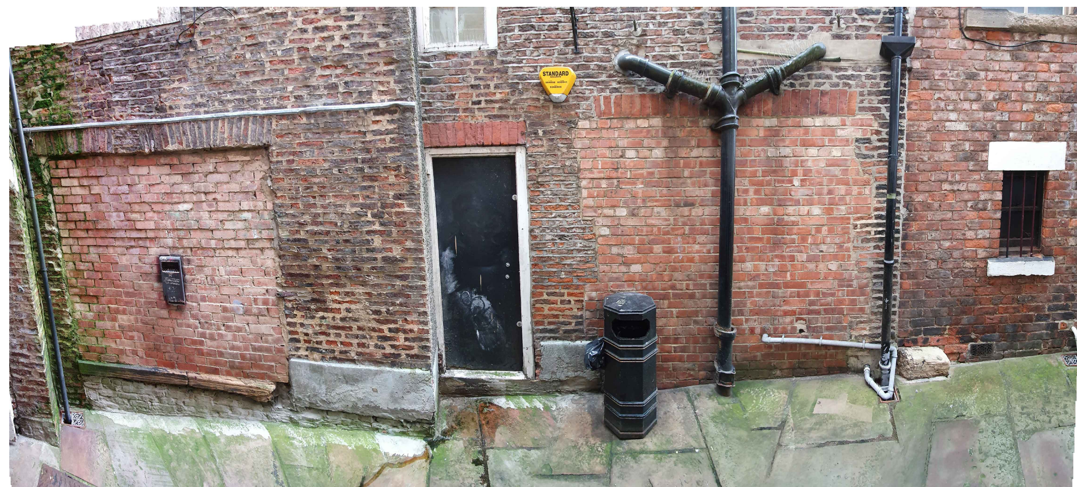
PHOTO (EXISTING) - ENTRANCE FROM HIGH ROW TO BUCKTONS YARD - BUCKTONS YARD NTS @ A1
