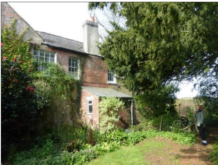
Fig.4 The rear wing with the sash window (left) which originally served the third bedroom. The other windows are later insertions.
