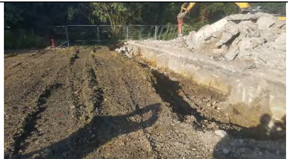
Area in SW (nr BH3) where slab is being lifted
