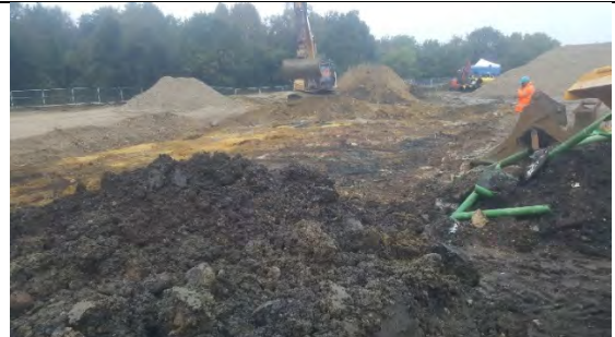
Area in SW being stripped of 'clean' material pre excavation to 2.5m depth. Background shows crushed concrete layer at surface
