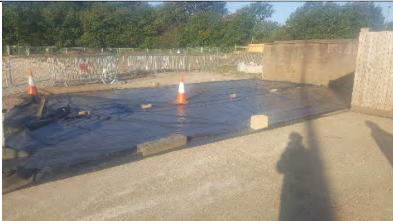
Bund area for water treatment
