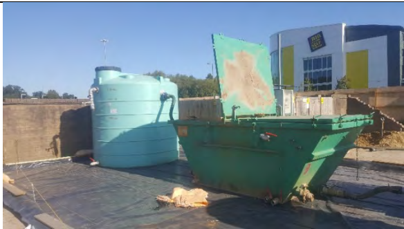
Water / oil separators
