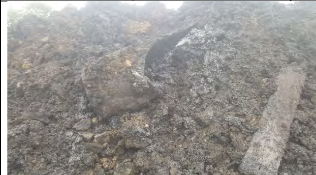
Relict gas works pipework pulled out, with tar like substance settled in base now oozing out
