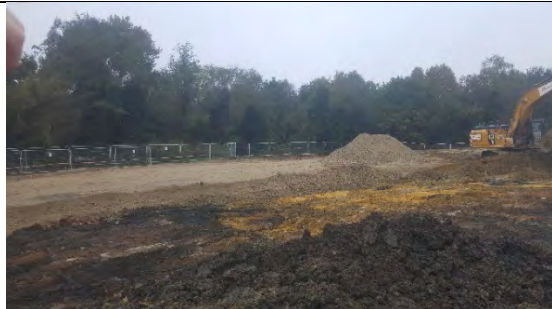
Area in SW being stripped of 'clean' material pre excavation to 2.5m depth. Background shows crushed concrete layer at surface
