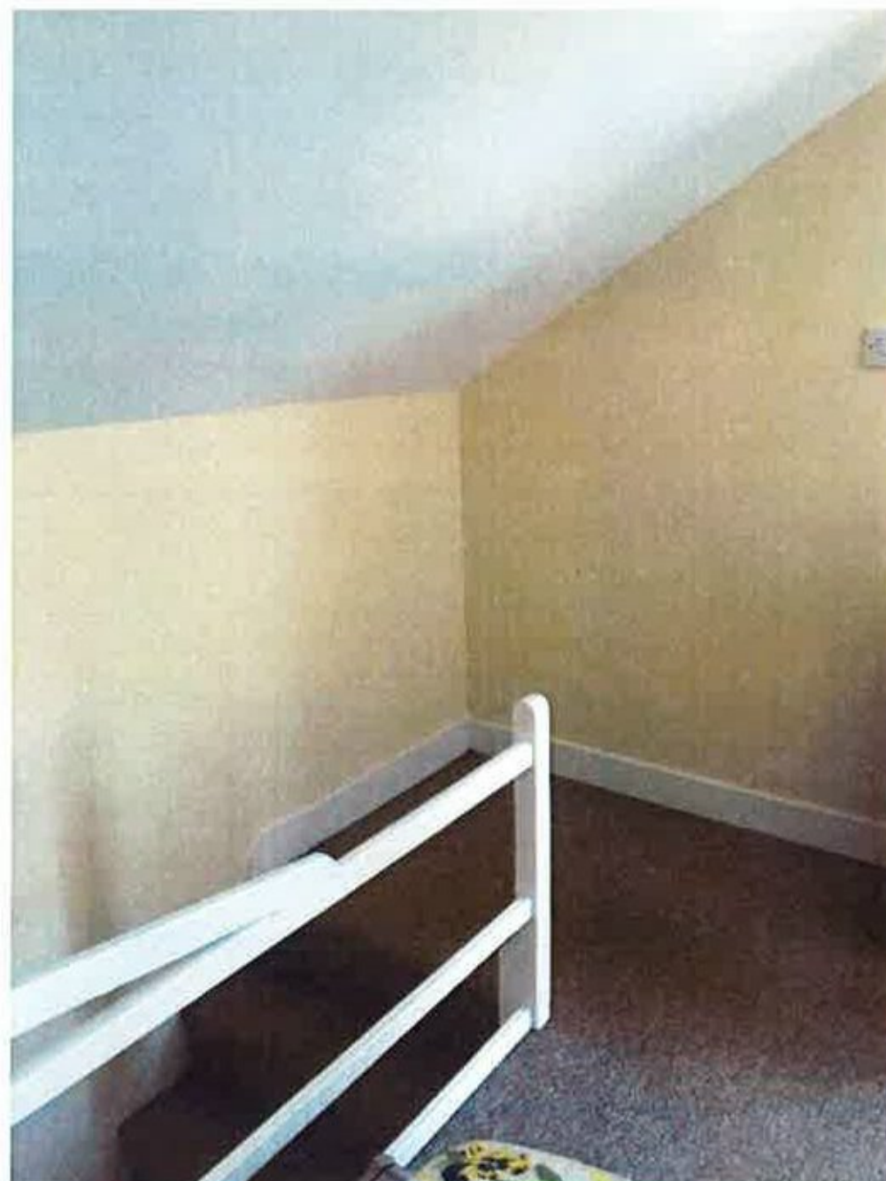
Low head room above the staircase.
