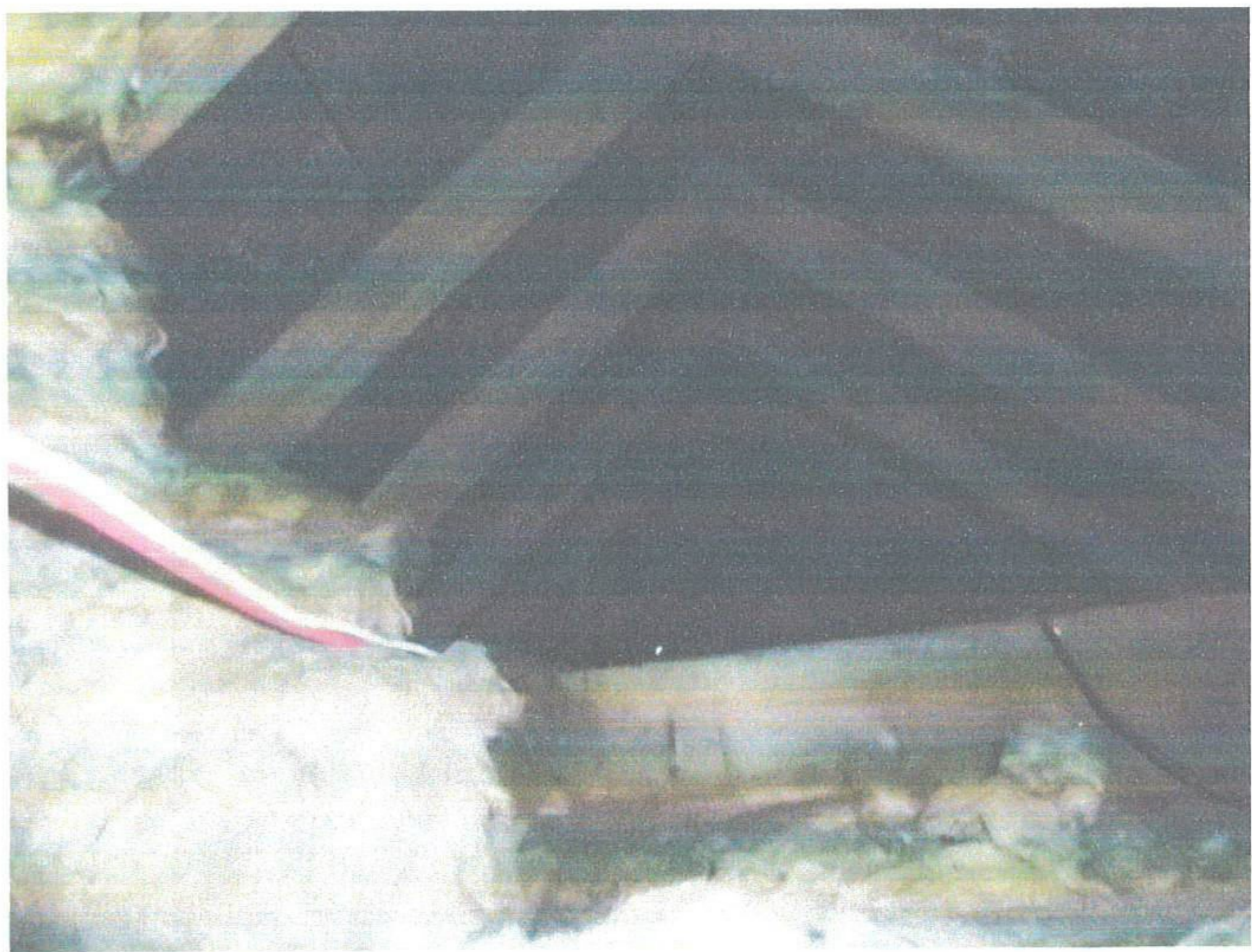
Plate 7. The roof void over the eastern wing viewed from the small pop hole
