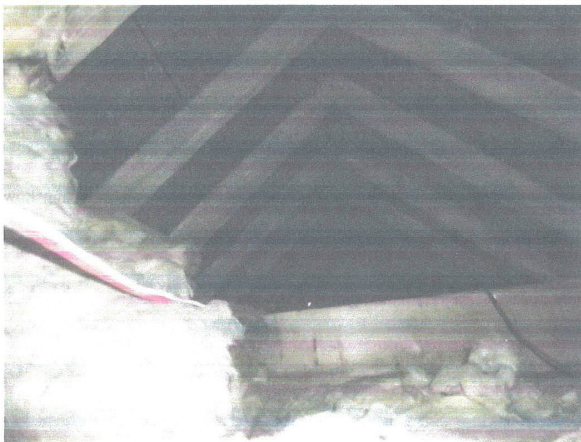
Plate 11. The roof void over the eastern wing viewed from the small pop hole
