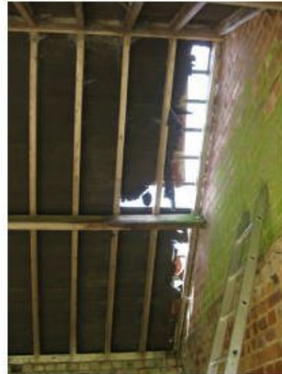
Photograph 2: Interior of the barn, showing gaps in the roof
