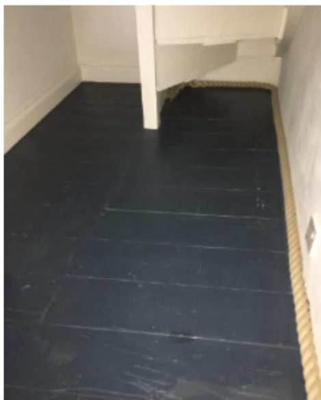
Ref Image 1 1 st floor landing, here you can clearly see the infill floor boards where the original staircase would have been.
