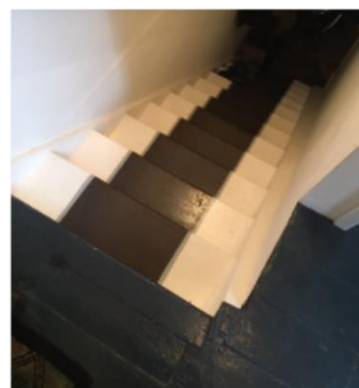
Ref Image 3 The current staircase which badly impacts the scale and proportion of both ground floor and 1 st floor rooms
