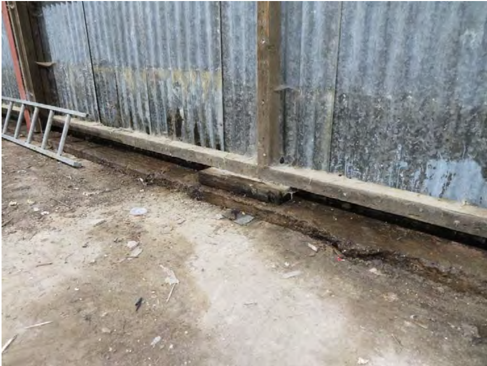
Photograph 17: Difference in levels between assumed original foundations and ground slab.
