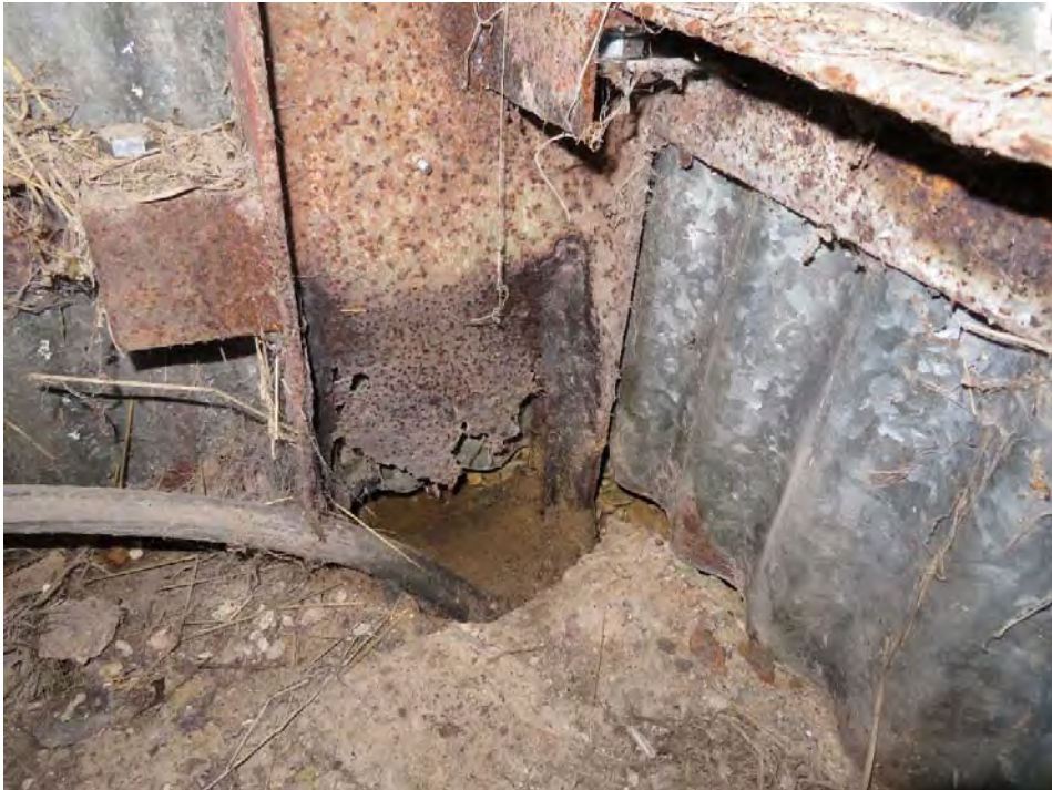
Photograph 7: Delaminated corner column – close up of Photograph: 6.
