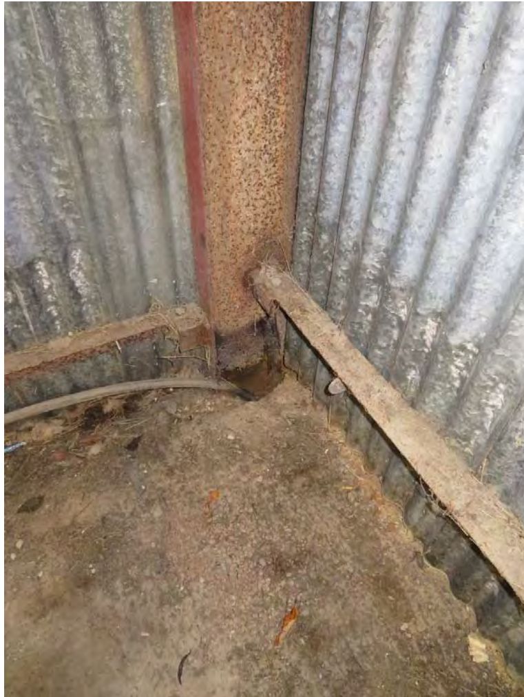
Photograph 6: Delaminated corner column – part of web is missing
