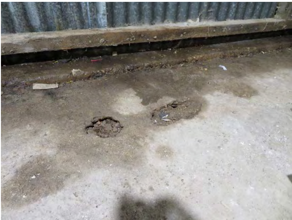
Photograph 18: Voids to ground slab.
