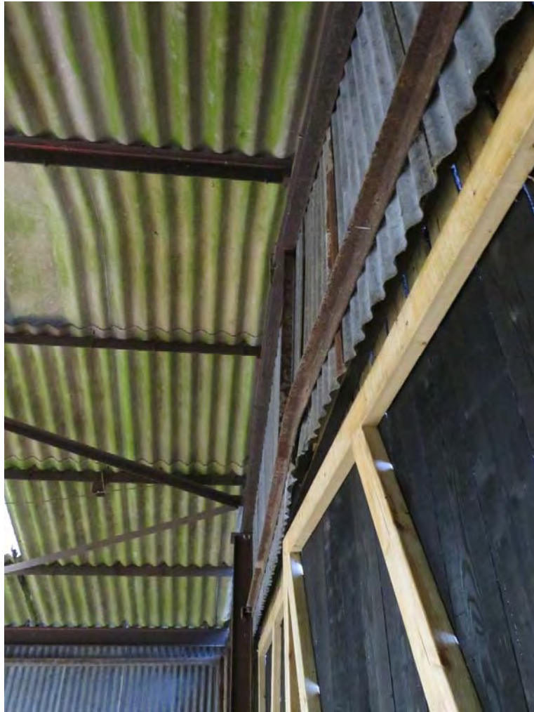
Photograph 4: Deformed/distorted steelwork over head of doors.
