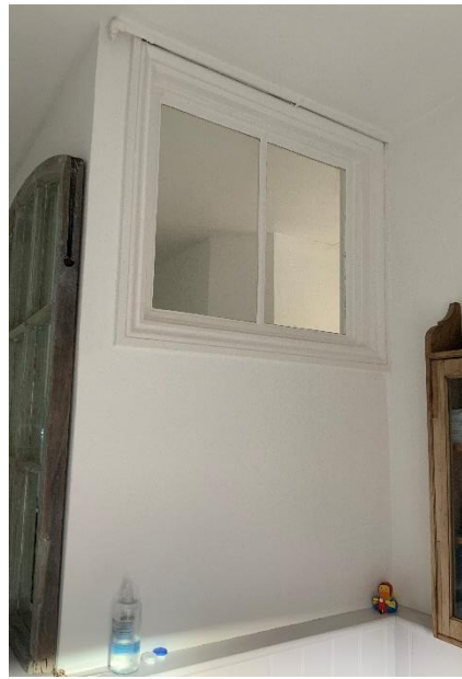
View of existing internal bathroom window from within the bathroom – to be blocked up
