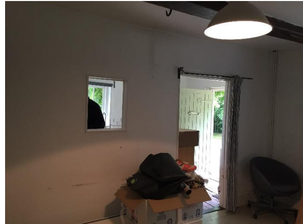
Internal ground floor annex wall between the kitchen area and living room – to be demolished
