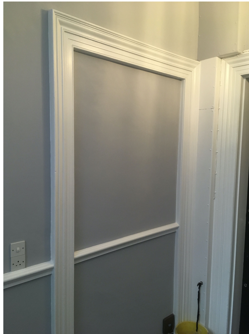
IMAGE 02 - BUILDING N.42 IMAGE SHOWING POSITION OF NEW ENTRANCE DOOR. THE NEW DOOR SEES THE RE OPENING AN EXISTING OLD BLOCKED DOOR. EXISTING ARCHITRAVE TO BE KEPT IN SITU.
