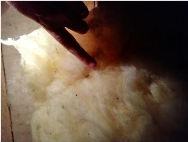
Figure 4 – Bat droppings within the former care home
