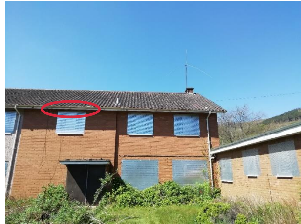
Figure 5 – Towards eastern aspect of two-storey section, and part of single-storey section (to right hand side) and known emergence point (x1)
