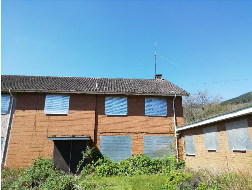
Figure 5 – Towards eastern aspect of two-storey section, and part of single-storey section (to right hand side)
