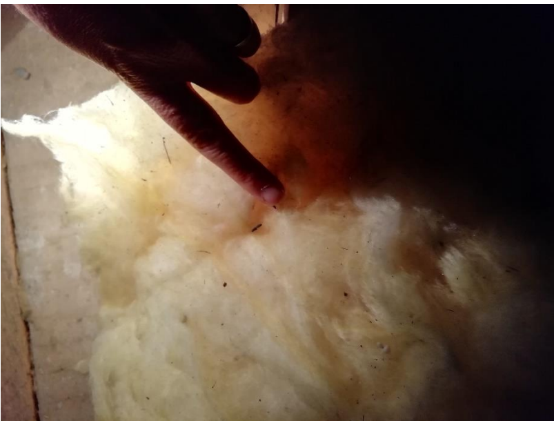
Figure 4 – Droppings found in roof void
