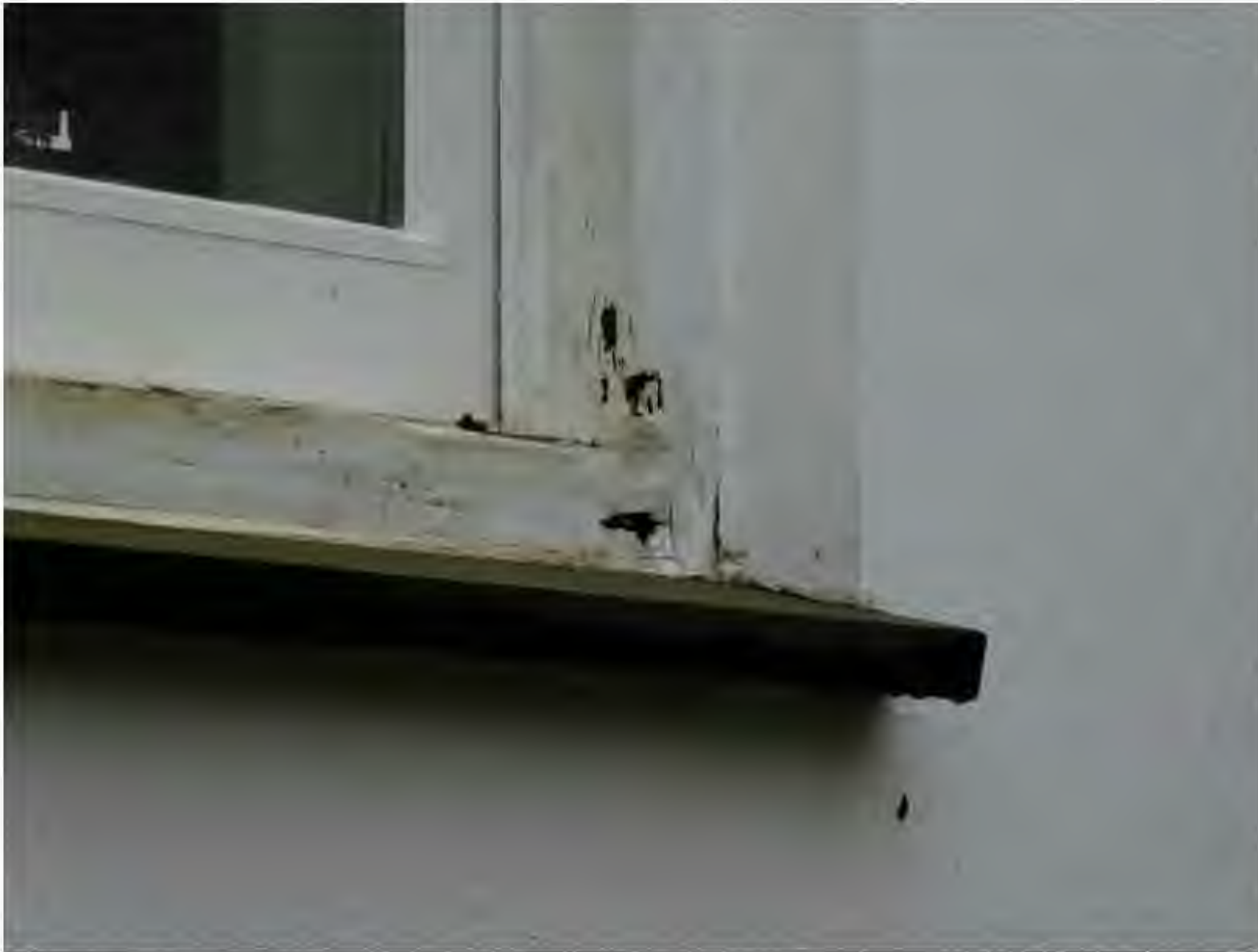
Example of Window Cill Decay
