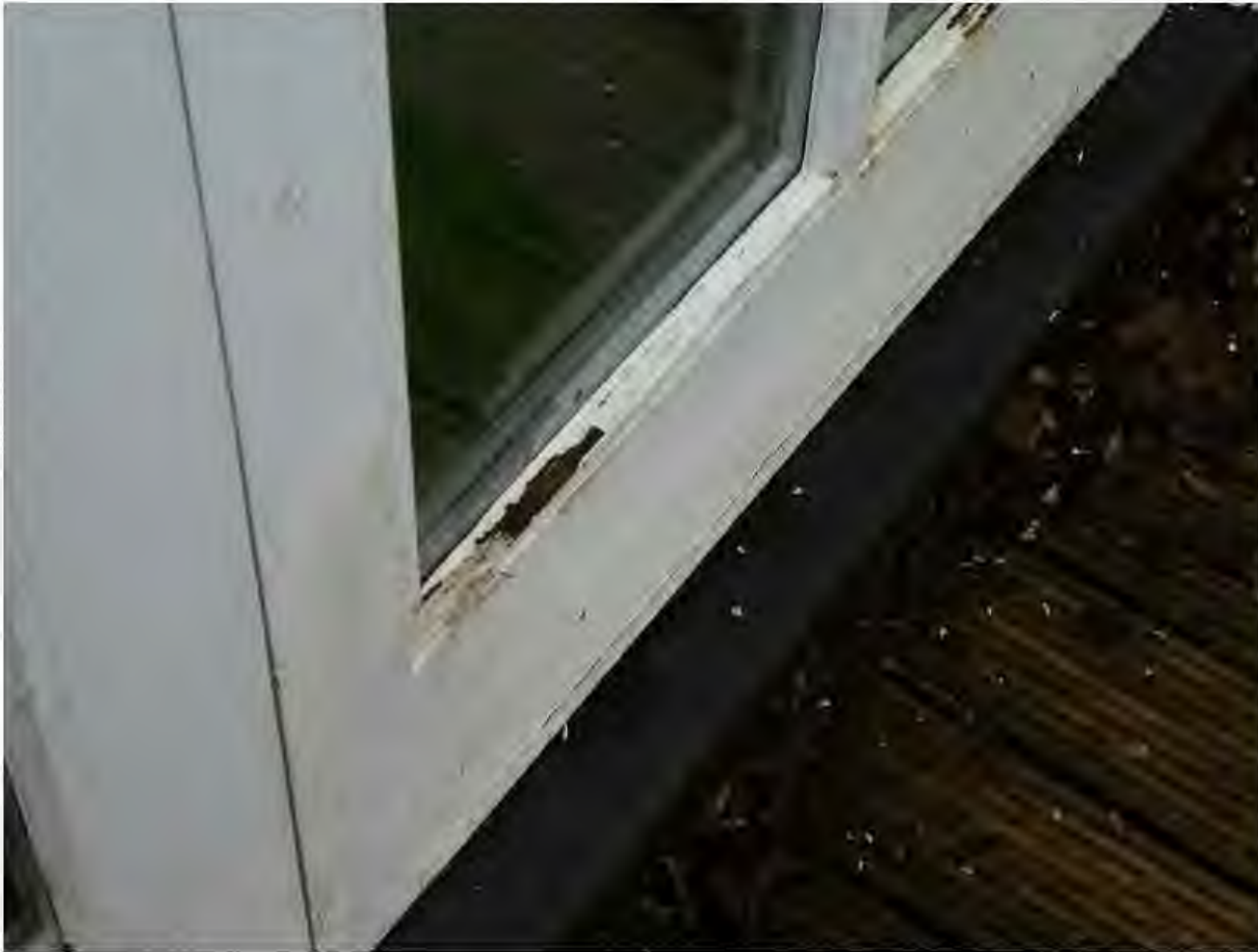
Example of Door Decay
