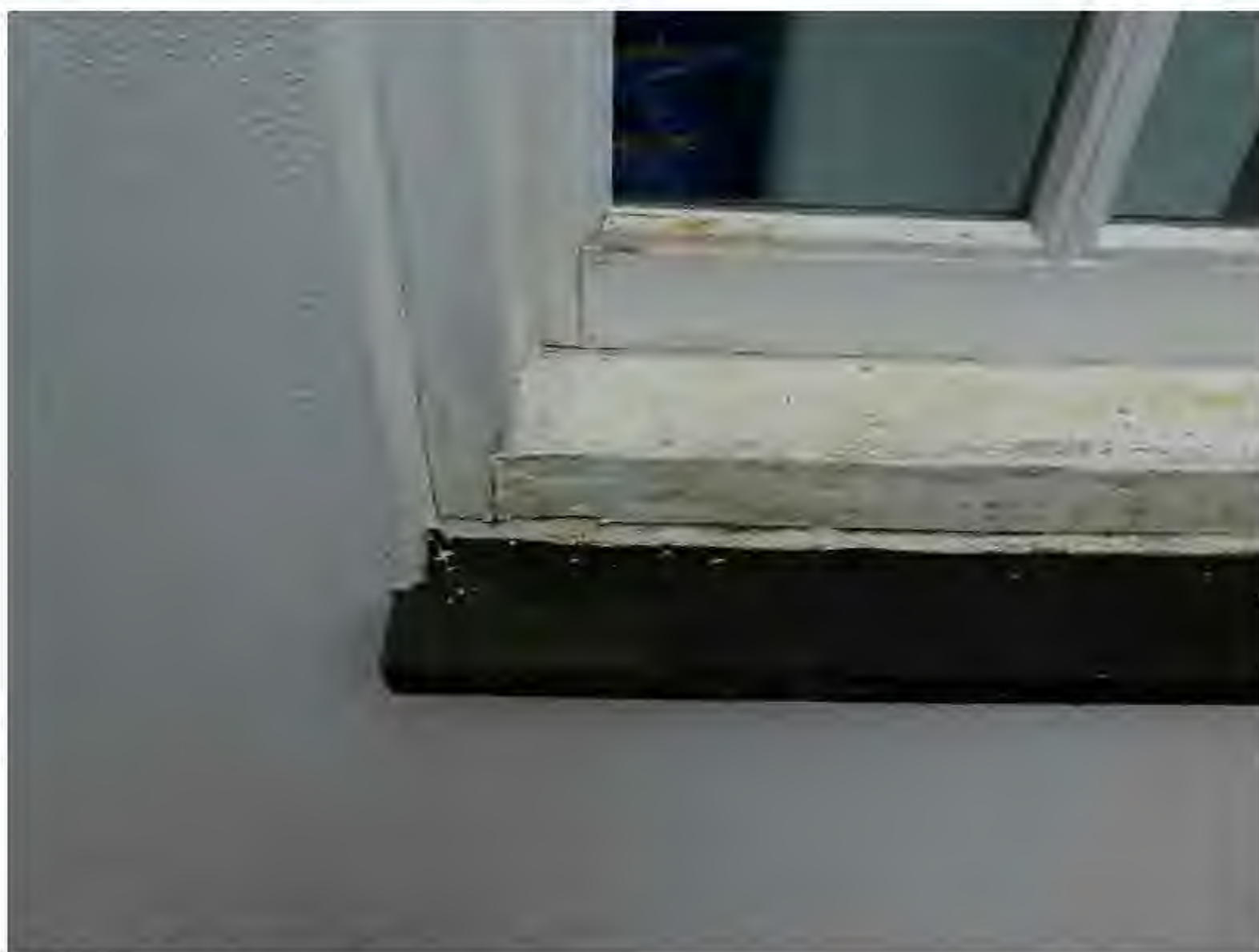
Example of Window Cill Decay
