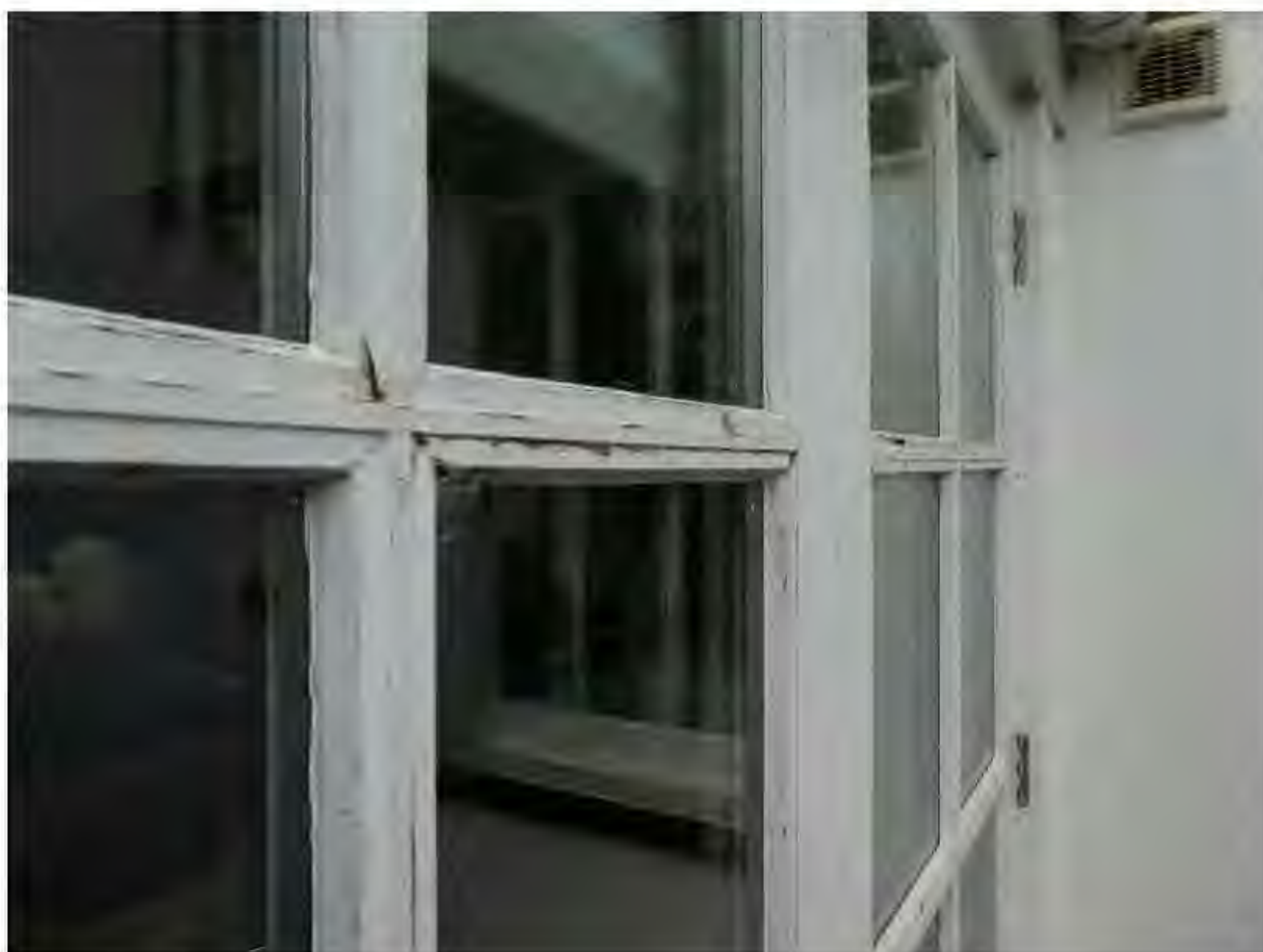
Example of Door Decay
