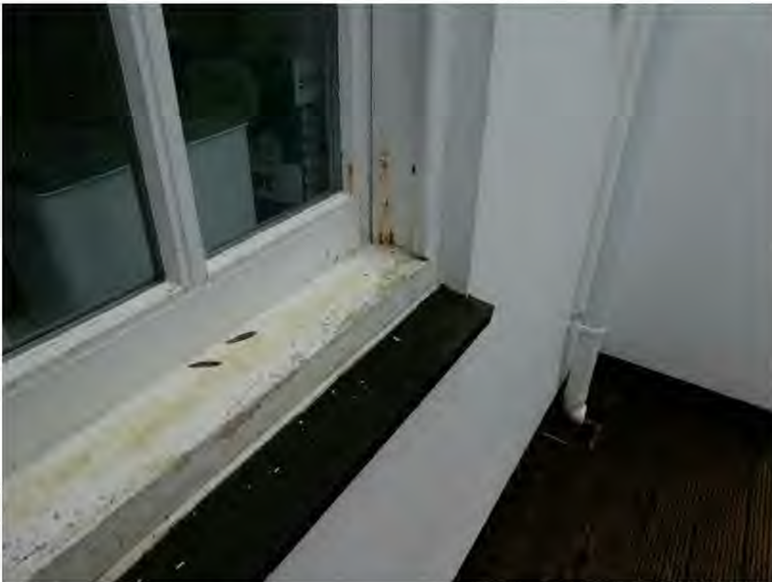
Example of Window Cill Decay
