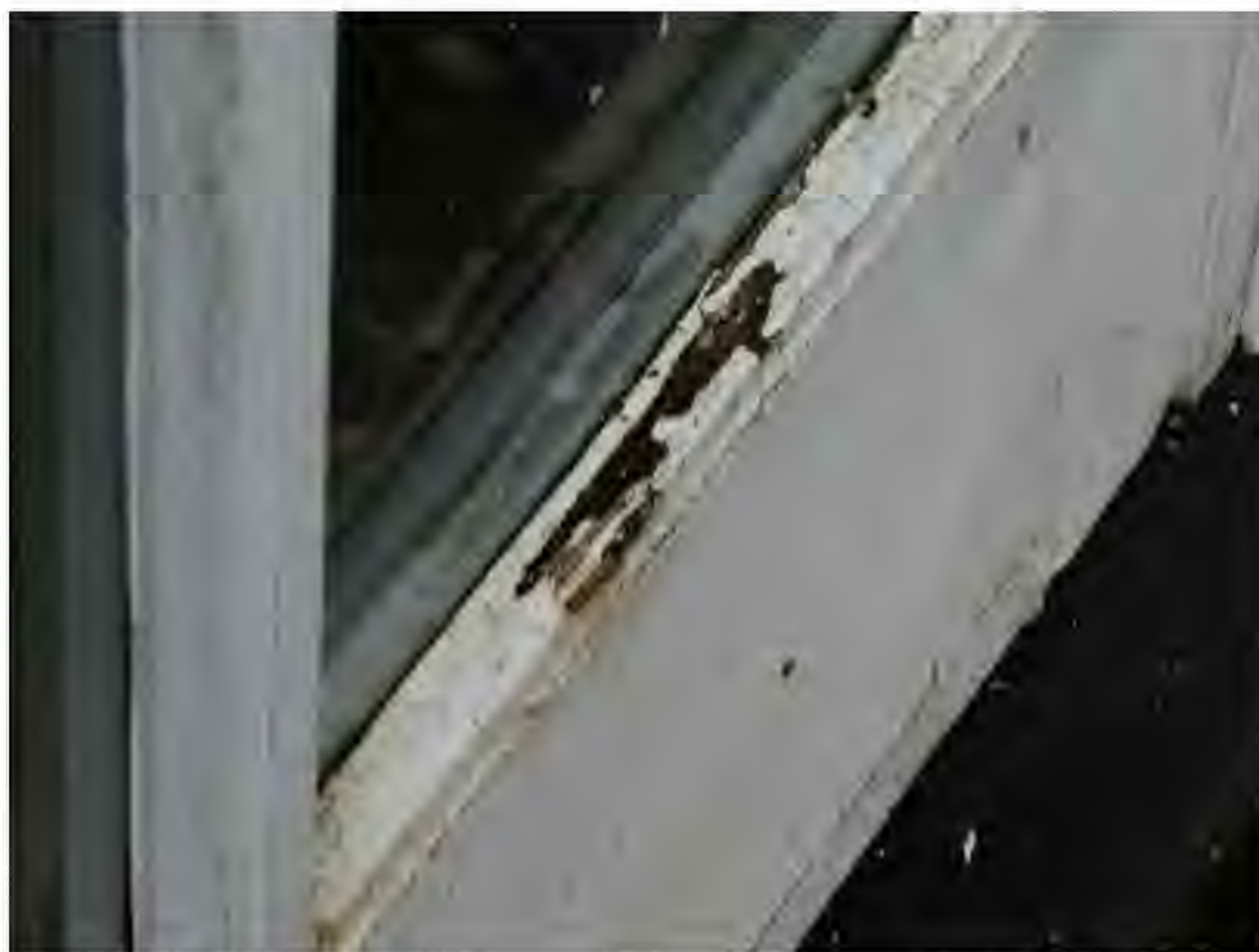
Example of Door Decay
