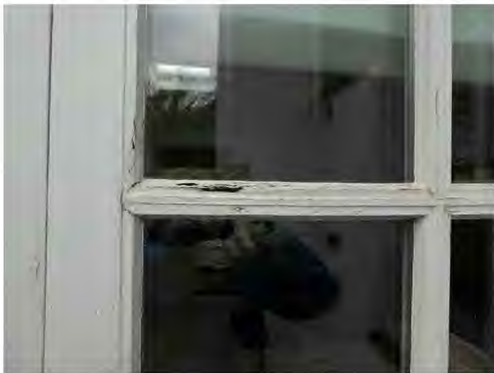
Example of Door Decay
