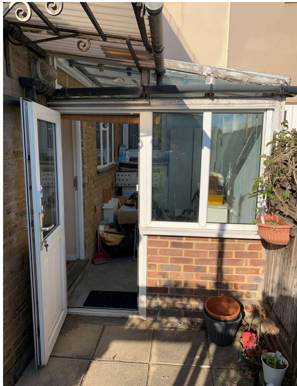
Photo 04: Rear view of the existing conservatory at Park road 37 at party wall with Park road no. 35.
