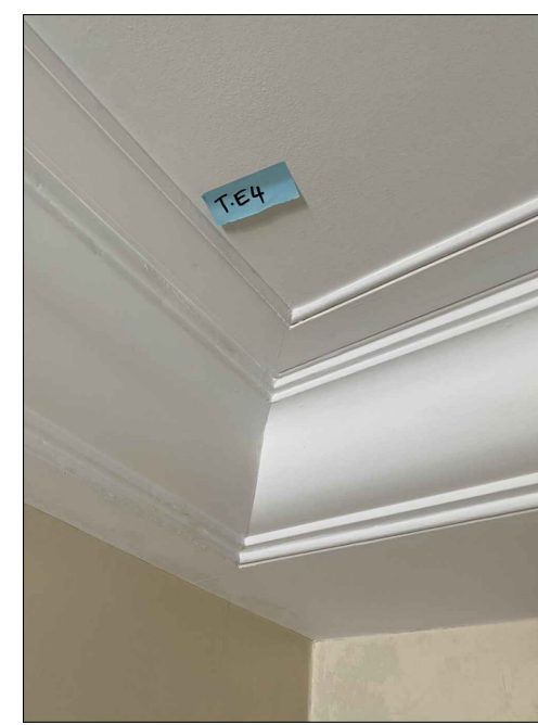
Existing (3F Guest bedroom T-E4) Coving to match and install in New Bedrooms T-04 T-06 T-07 and Hallway T-01 and Lobby T-09
