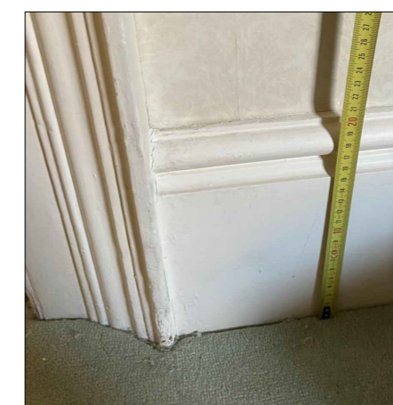
Existing 1F Skirting (Petit Salon F-05) to be fully refurbished
