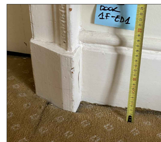
Existing 1F Skirting (Hallway F02) to be fully refurbished
