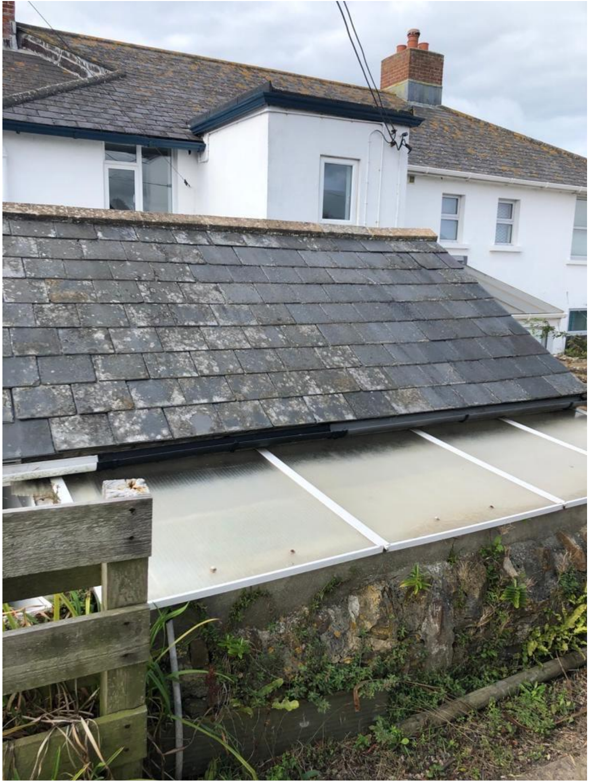
Boot room roof (foreground) and north side of roof to 6 Coastguard Cottages
