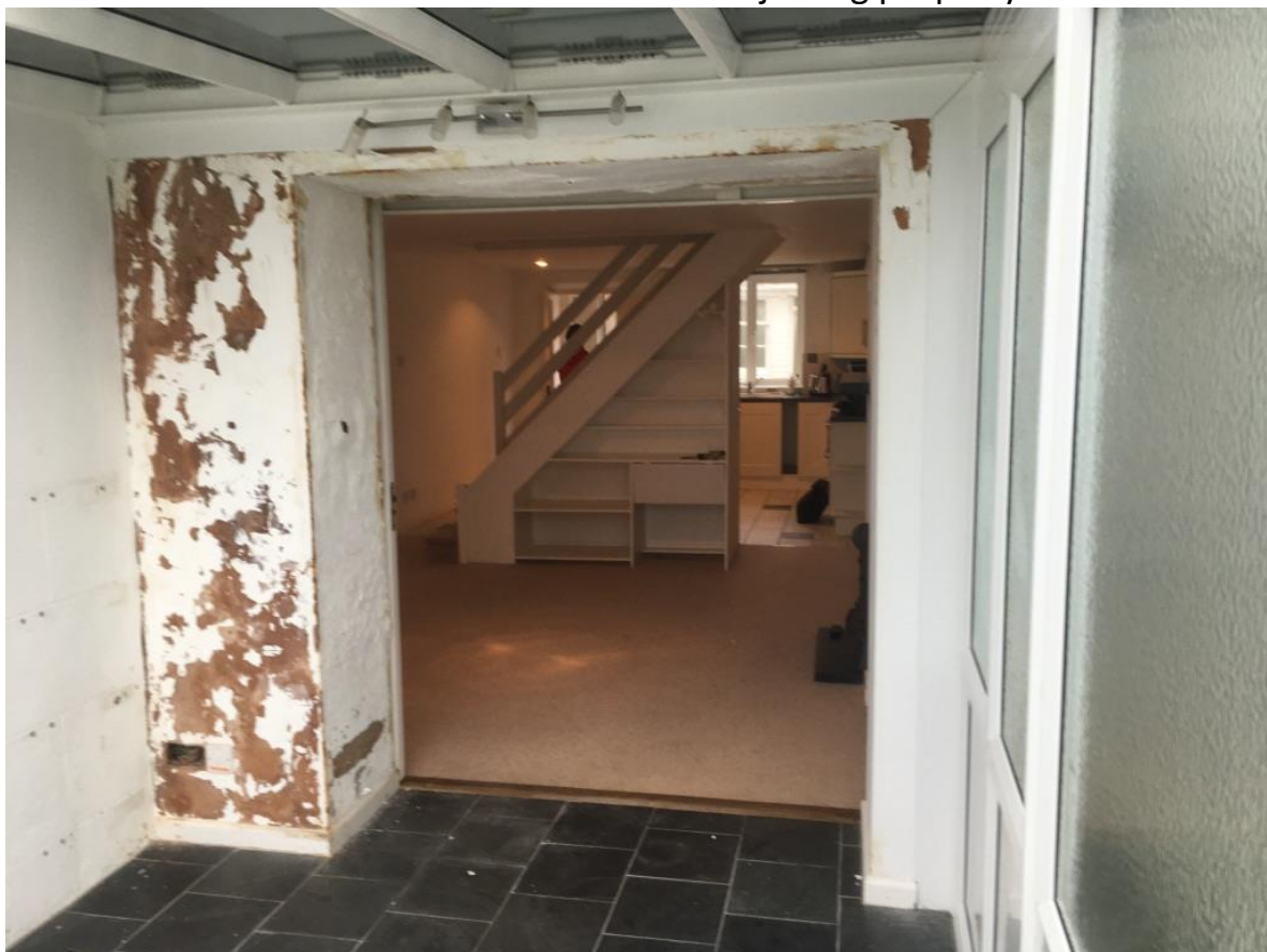
Water ingress to south facing wall in conservatory
