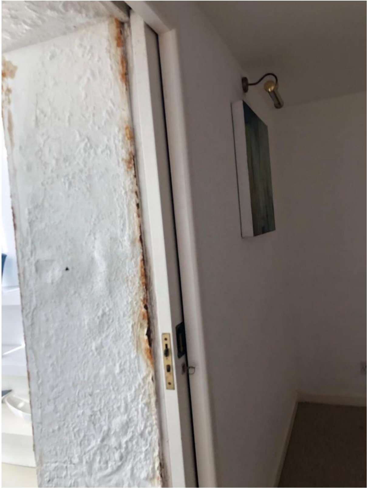
Water damage to reveal in south wall between conservatory and living room.
