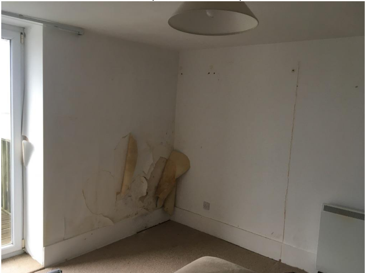
Water damage to external wall to bedroom 1
