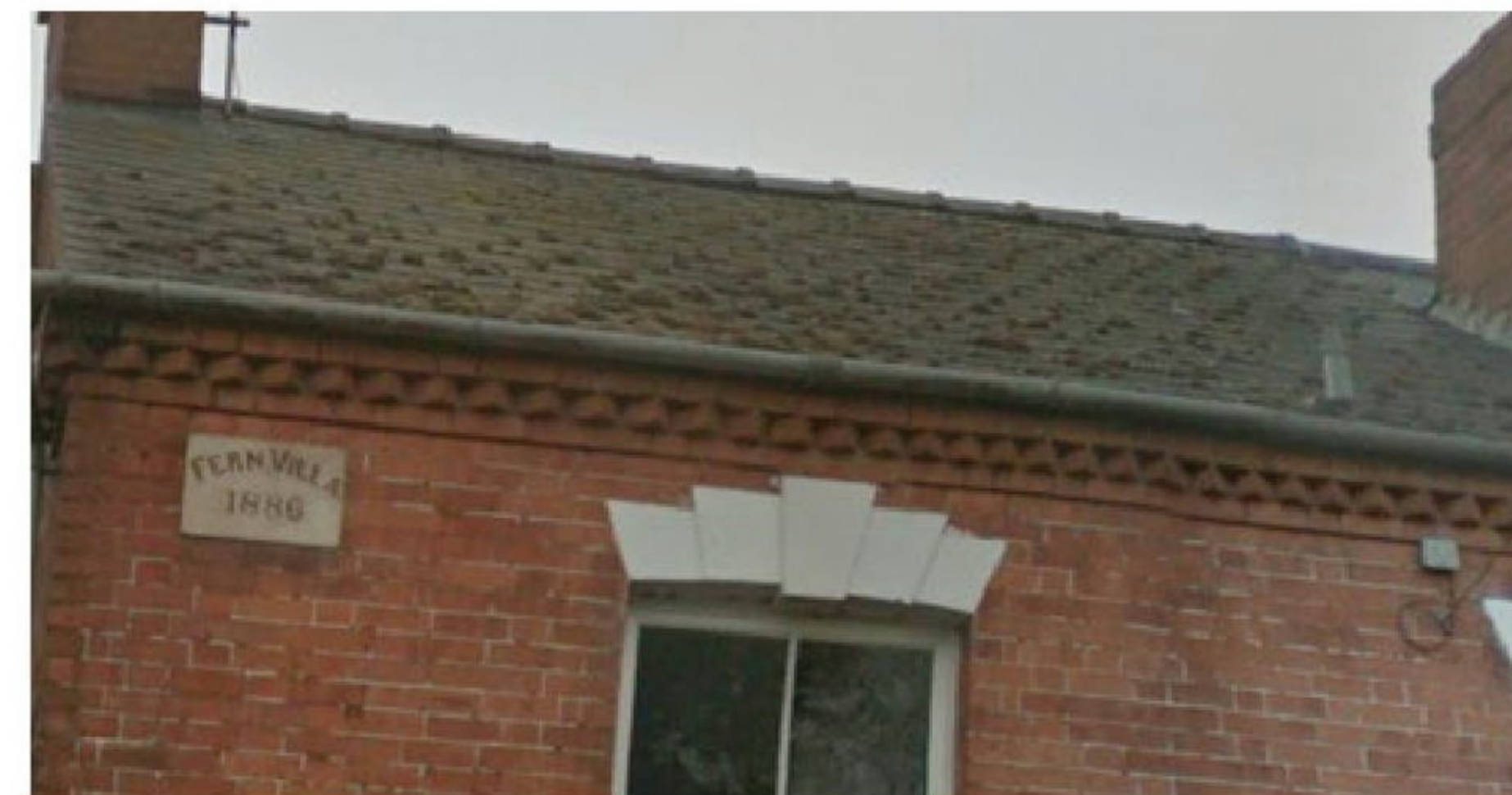
Window head detail and dog tooth brick coursing on property adjoining Lion House. (45)
