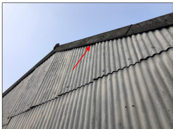
Photo 15: Gaps between barge board and cladding
