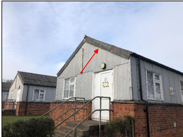
Photo 12: Gaps under barge board
