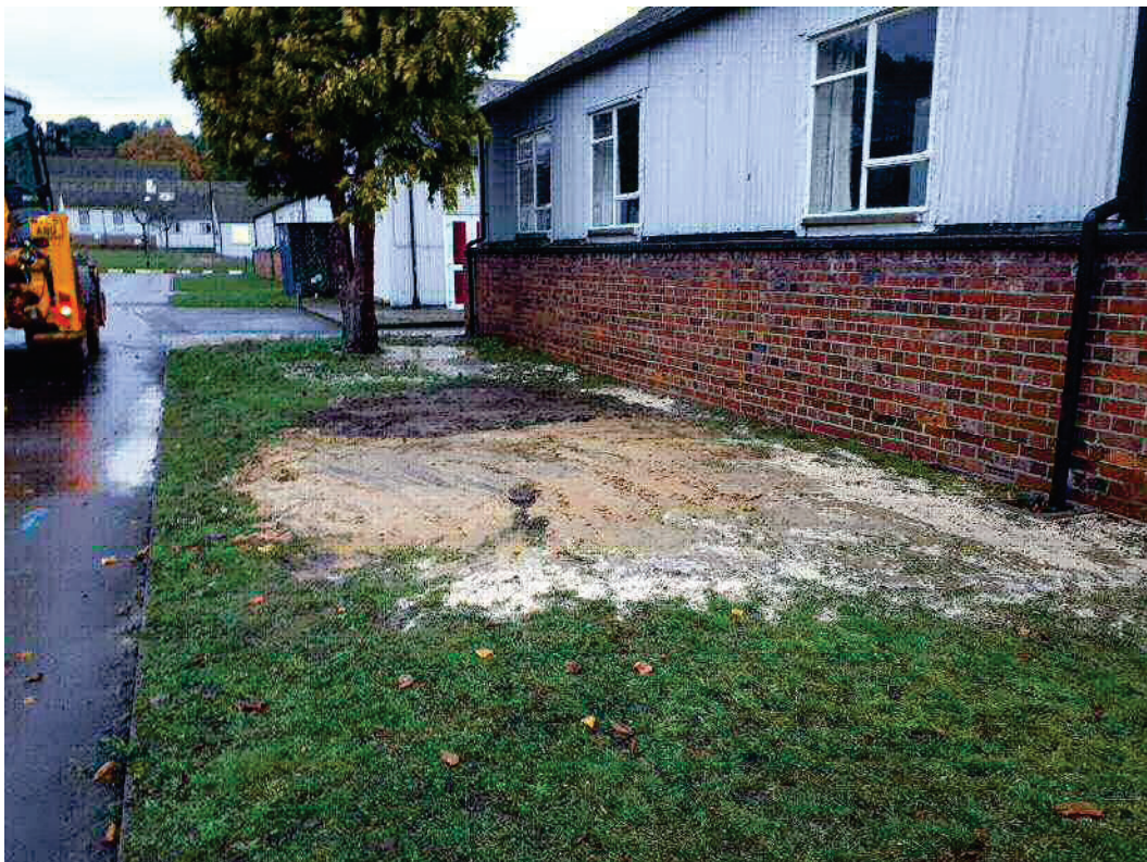
Photograph 2: View of TP01 after reinstatement, located at the centre of the site.
