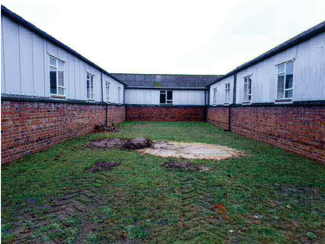
Photograph 1: View of one of the existing single storeys structures. Photo taken across TP03 located south-east of the site.
