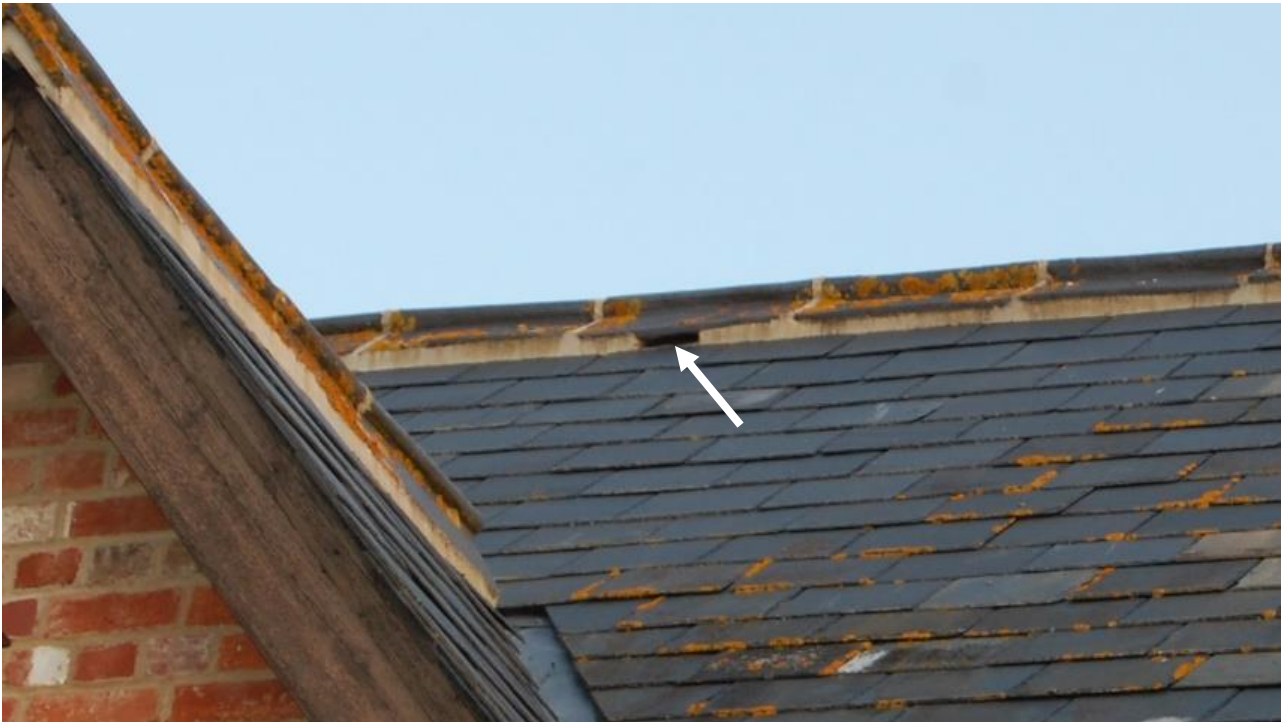
Figure 2. Detail of a roof showing a bat ridge tile (indicated by the arrow) incorporated within a slate-tiled roof.
