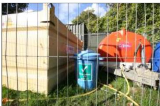
Pollution image 1: Where fuel or other chemicals are stored on site, it is now standard practice to have emergency spillage kits available to restrict the environmental impact of accidents.
