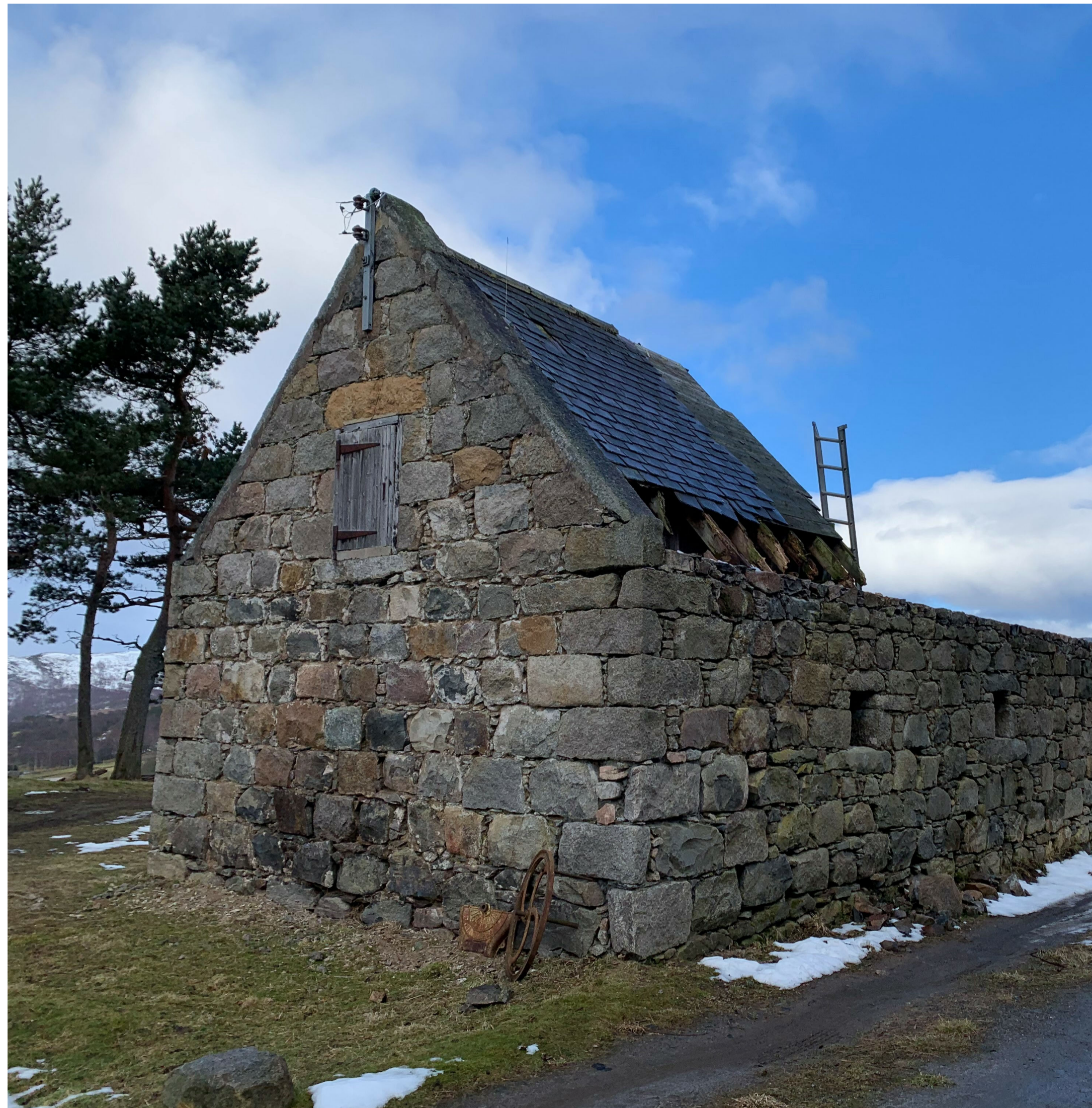
Taken 03.03.2020 North East Gable Steading after roof collapse
