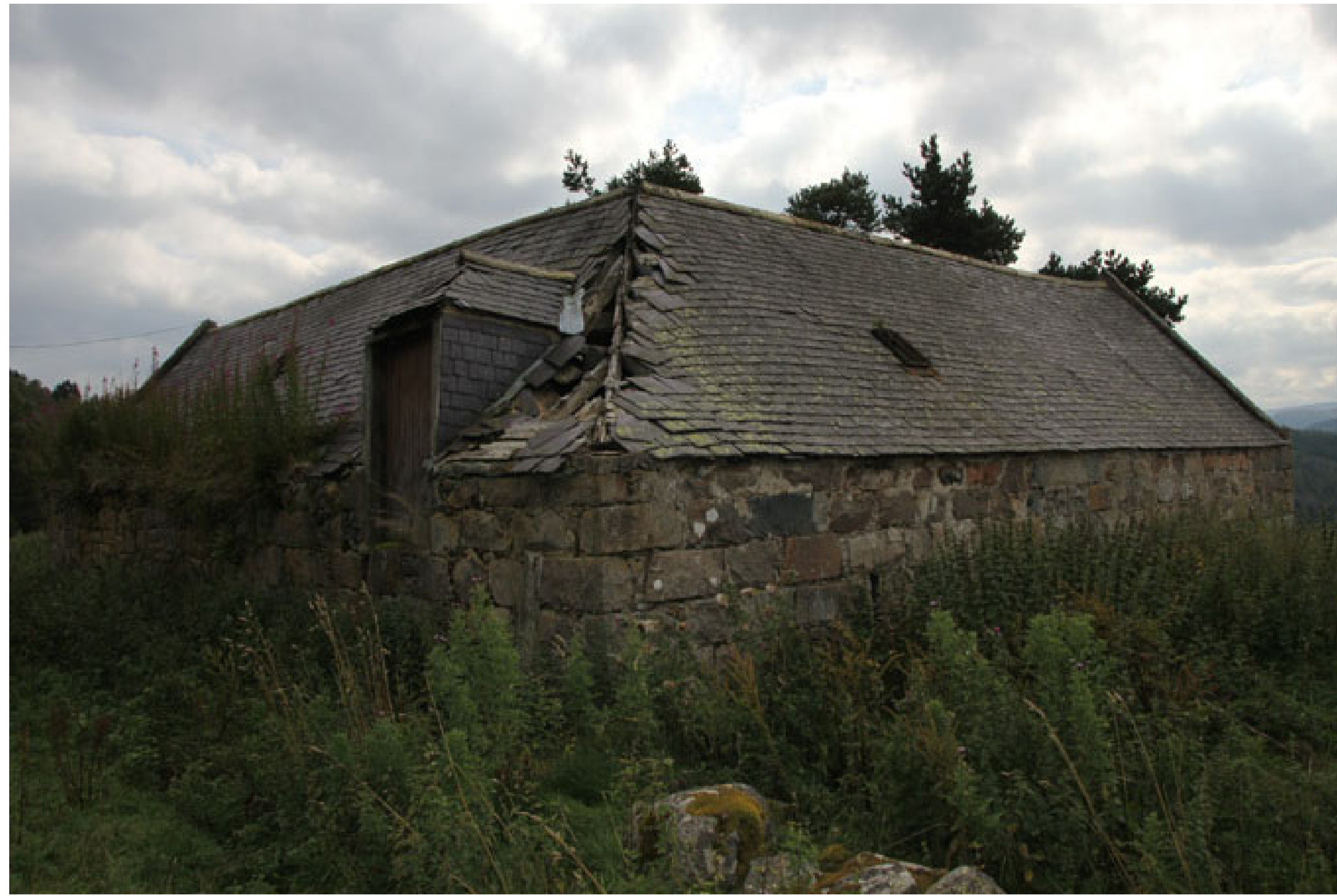
Taken 18.12.2011 North West corner Steading prior to complete collapse of roof
