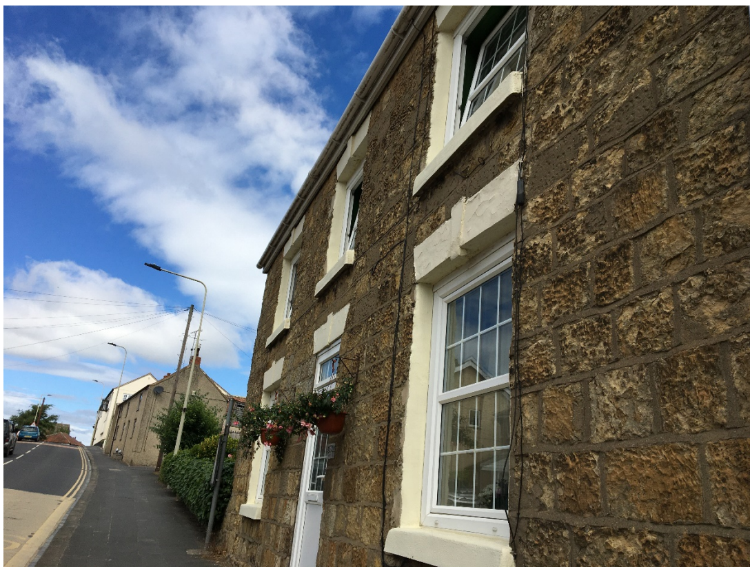
Plate 19 Close up of detail of flat arch with keystones on a historic building on Main Street – replacement uPVC windows are a slight detracting element.
