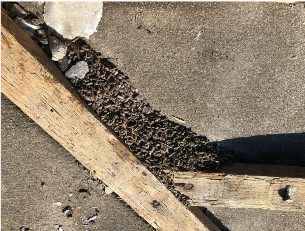
Figure 6: Example of bat droppings between slates (removed) and roof underlay, next to a roof valley.
