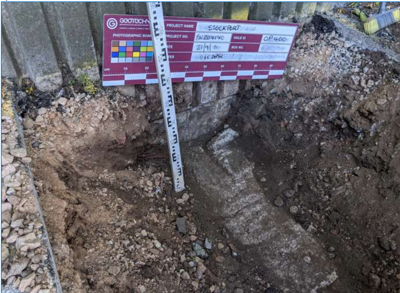
Figure 2 - OP400 excavated at the western end of DBRW (Swain Street end). Extent of excavation limited by kerbs.
