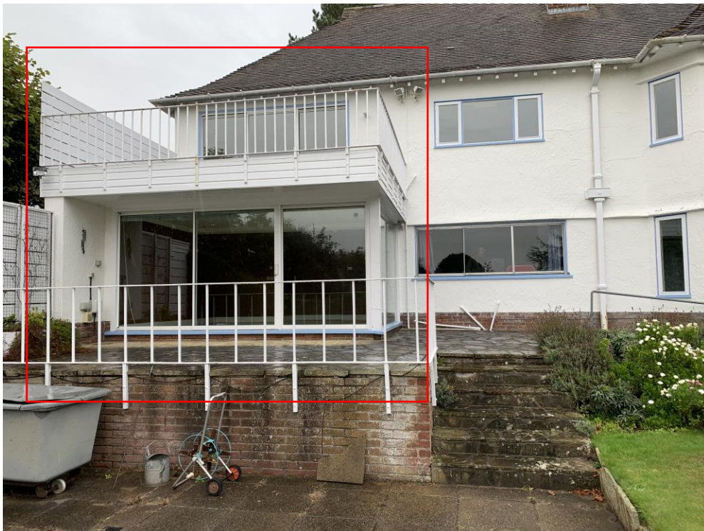
Rear elevation lounge and roof terrace to be replaced with new extension on existing footprint. Image 1 of 2 Nov 2020. The replacement of this existing and poorly constructed extension with a sympathetic, contemporary new two storey extension
