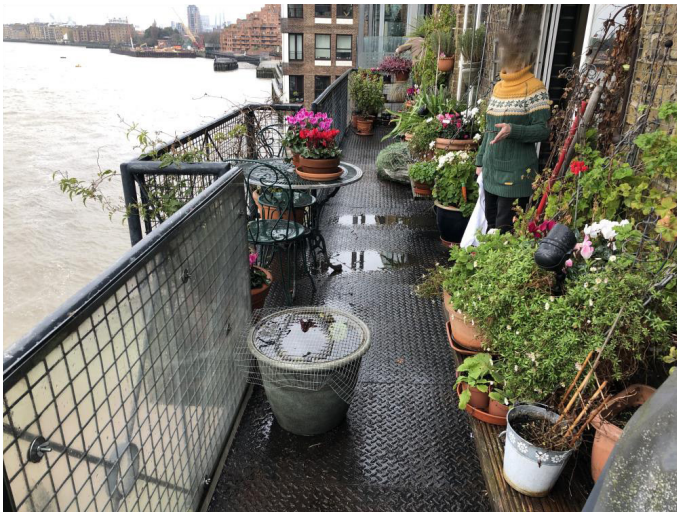
IMAGES FROM STRUCTURAL ENGINEER'S CONDITION REPORT
