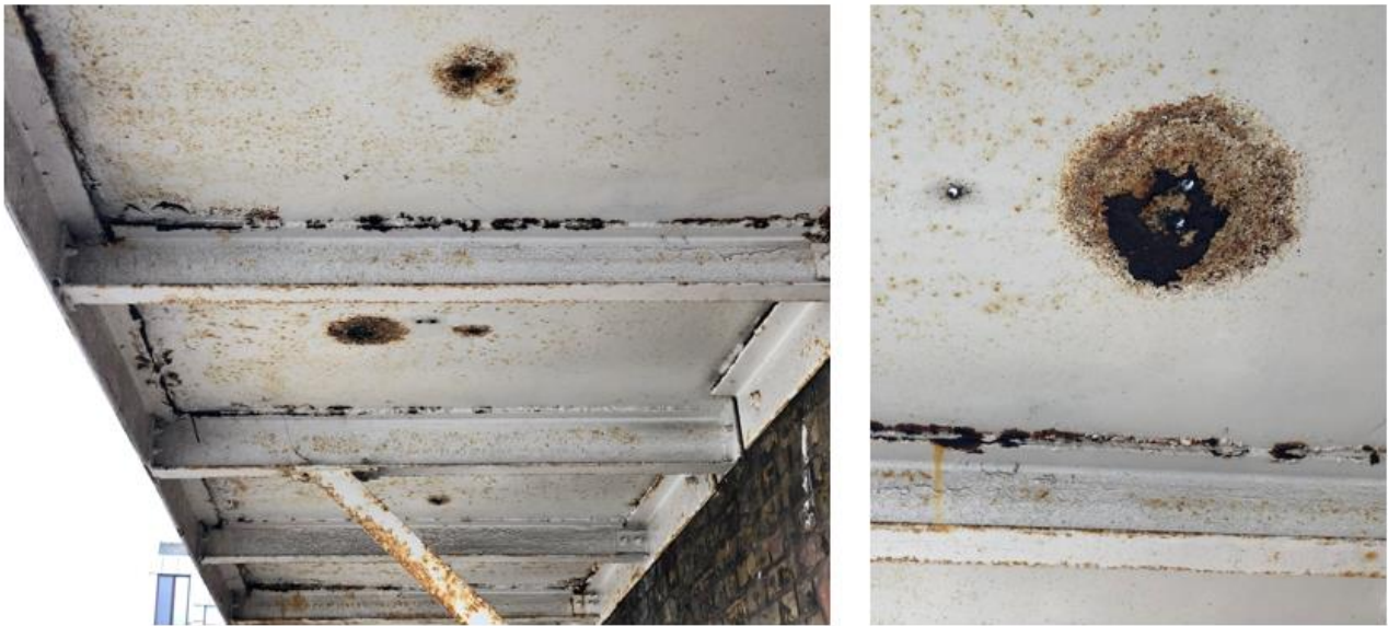
Figure 8 - Underside of fourth floor deck and drilled holes
