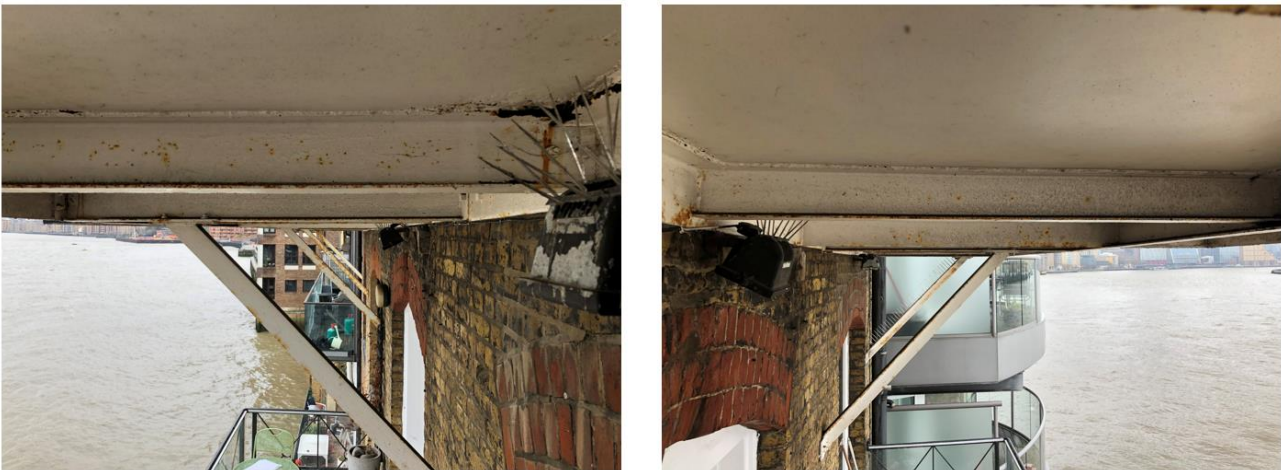
Figure 14 - From the double door access point, towards the West (Left) and towards the East (Right)
