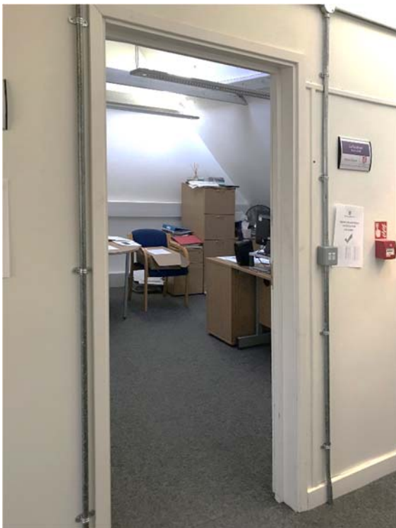
Figure 15 (above left). Looking from the Landing into a typical Office, showing the 2013 continuous floor finish, raised door heads and wall linings. The floor falls towards the desk and far corner.
