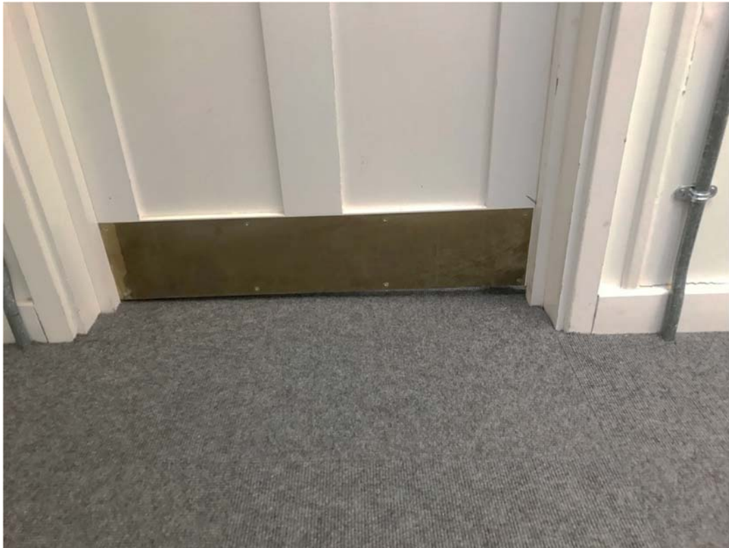
Figure 16. Showing typical gap below the fire door resulting from the sloping floor. This comprises carpet on a plywood underlay, covering the floorboards.
