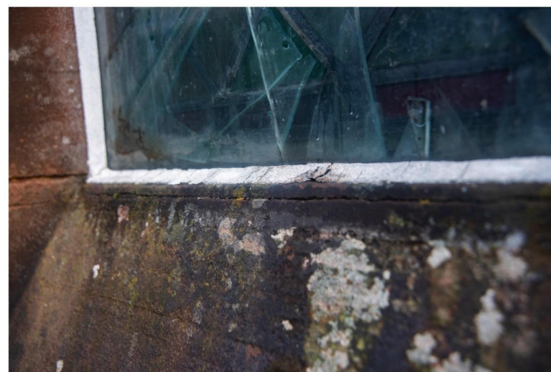
D) TYPICAL CRACK AT STONE CILL
