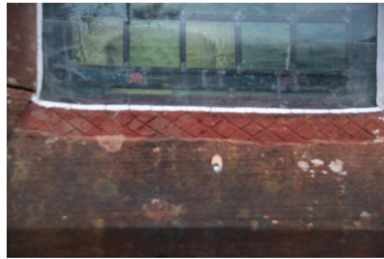
E) POOR PREVIOUS REPAIR
