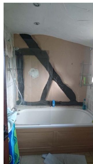
Evidence of A Frame in rear upstairs bathroom
