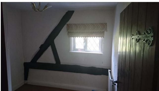
Evidence of A Frame in rear upstairs bedroom
