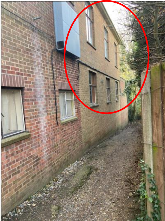
Existing windows (note, view to side of school) (windows circled are being replaced)
