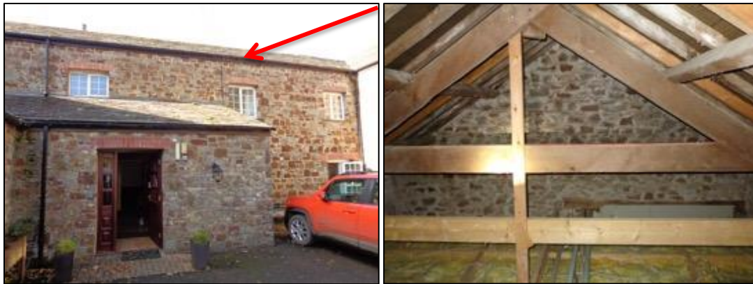
Figures 3 & 4. Bat access points along the eastern elevation wall-top will be retained and unaffected by proposals [left]; interior view of roof void
