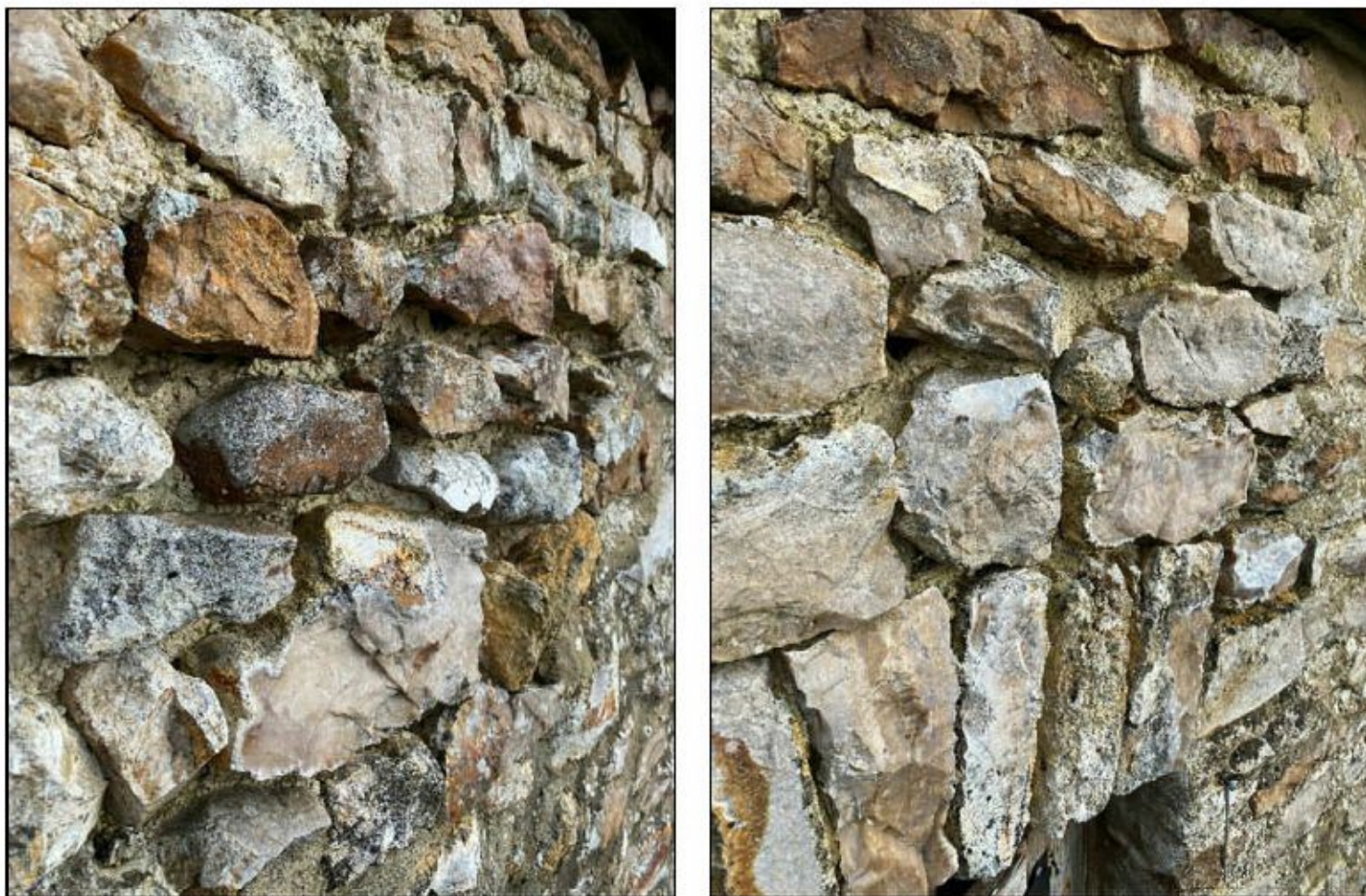
Image 7 – Some areas of the exterior wall requiring repointing to prevent further deterioration.
