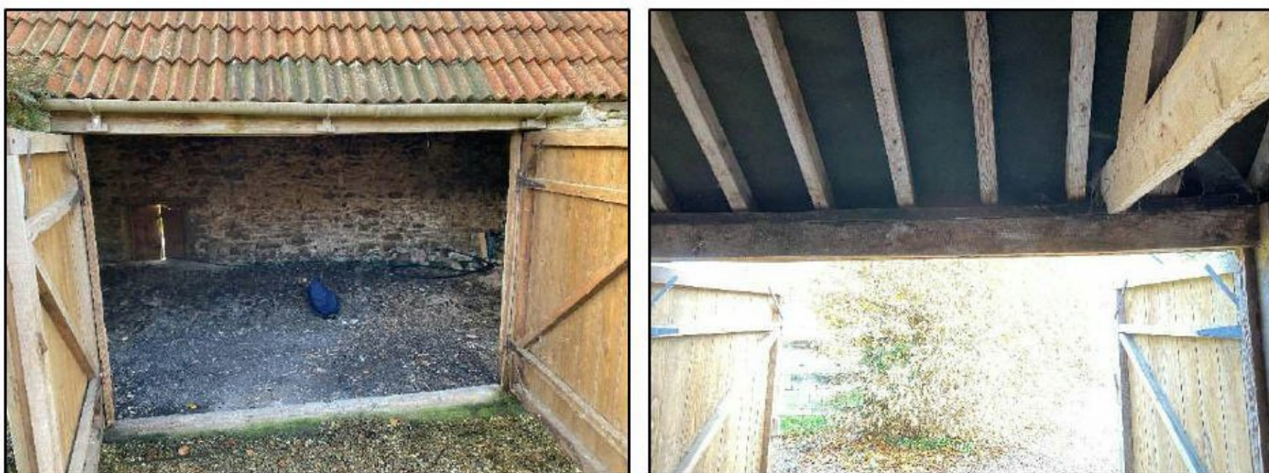
Image 2 – Double door access (left) and roof truss bottom chord bearing on timber lintel over access doors (right).
