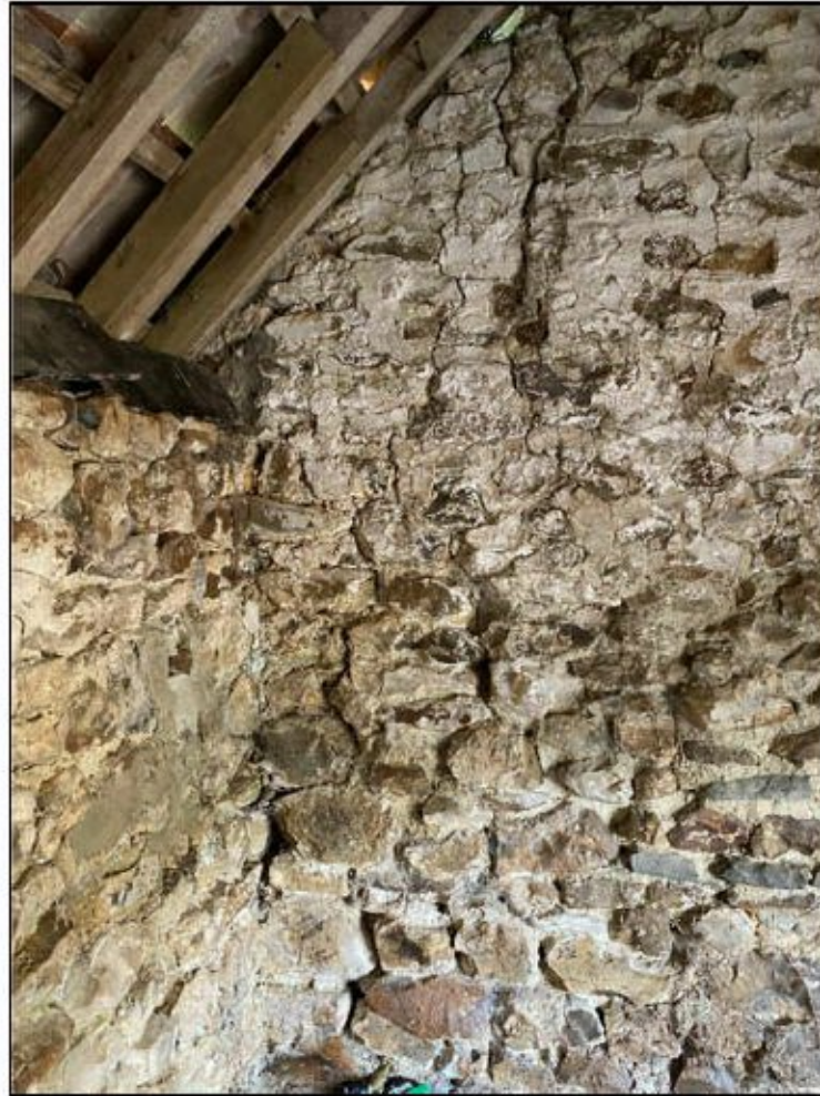
Image 4 – Minor cracking in the West corner of the building under the purlin bearing.
