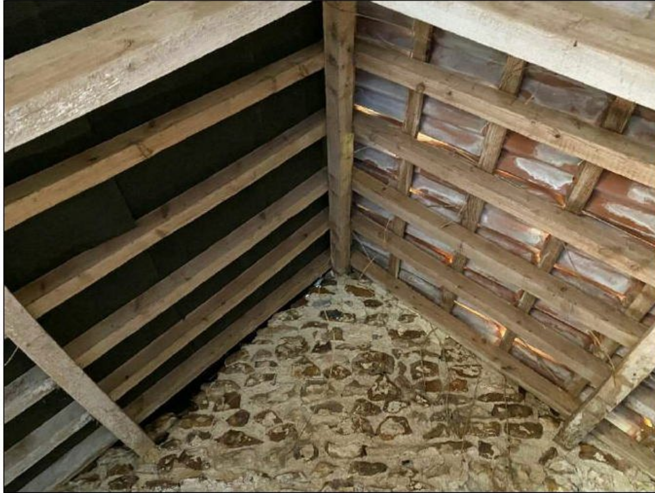
Image 3 – Evidence of roof felt installed on the North Eastern side of the roof only.
