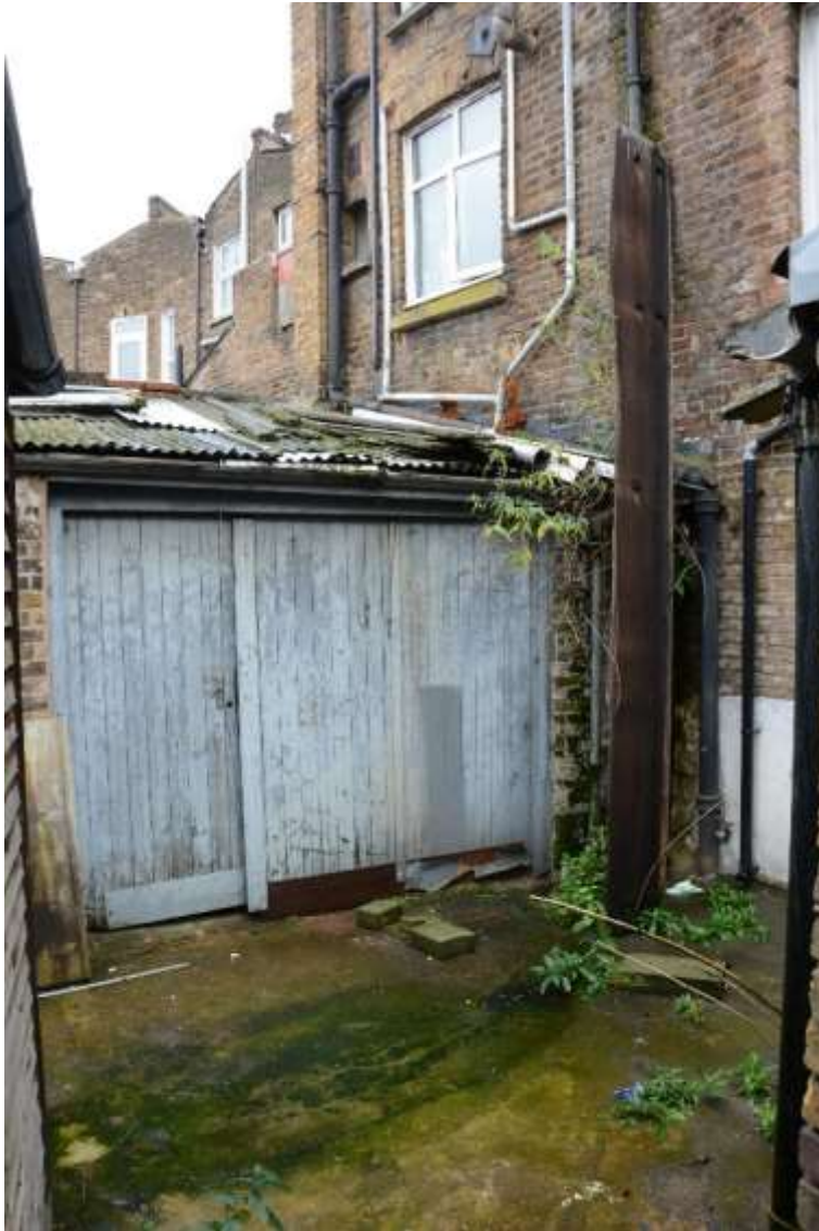
Figure 27: 8: Rear yard of No.10. No.6 is just visible in the top left corner of frame. Facing E.
