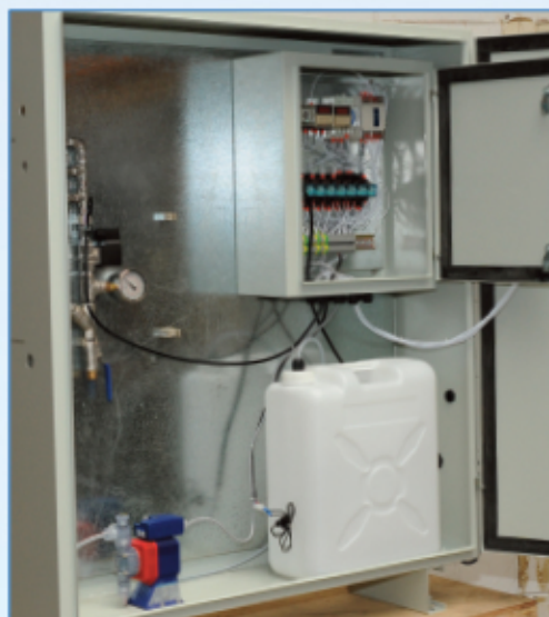
INTERIOR OF AUTOWASH CABINET
