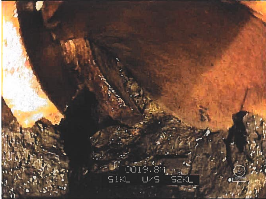
5, 00:04:31, 19.80 m Collapsed drain or sewer
