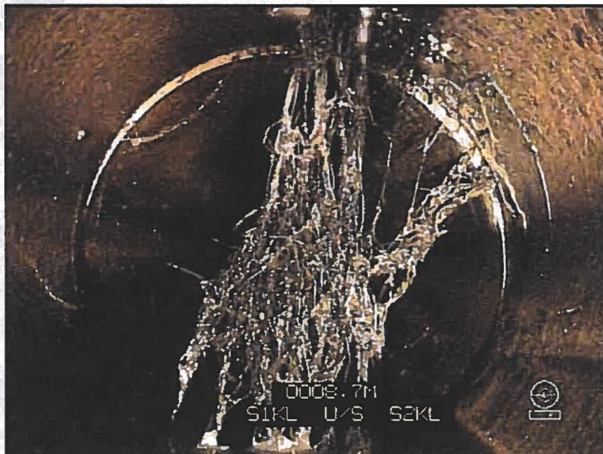
2, 00:02:22, 8.70 m Roots, fine at joint
