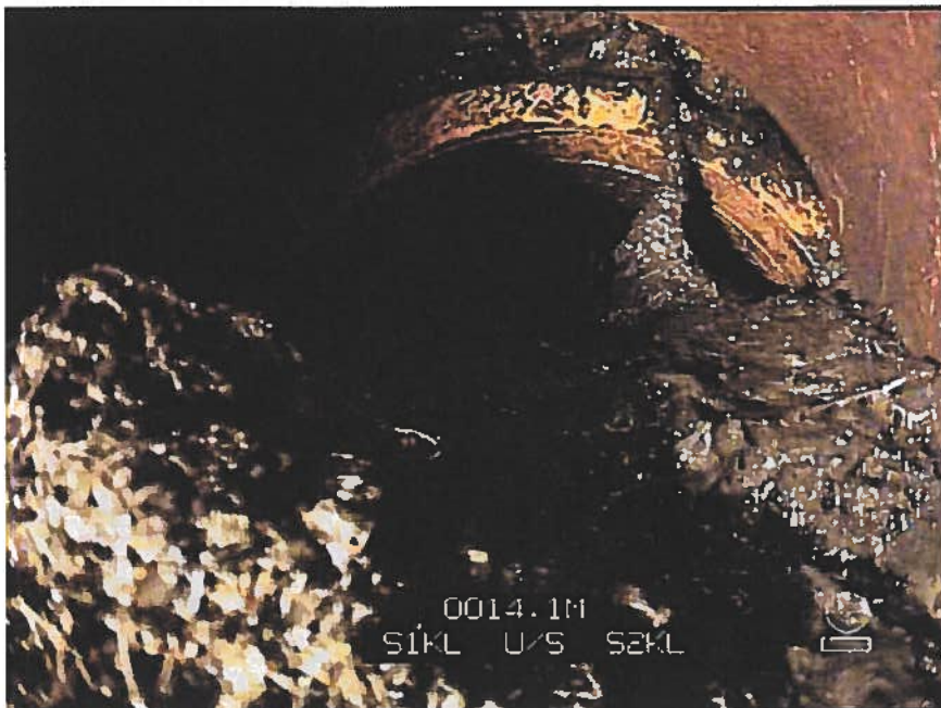
3, 00:03:33, 14.10 m Defective junction, blocked at 10 o'clock, diameter: 150mm, Roots in JN
