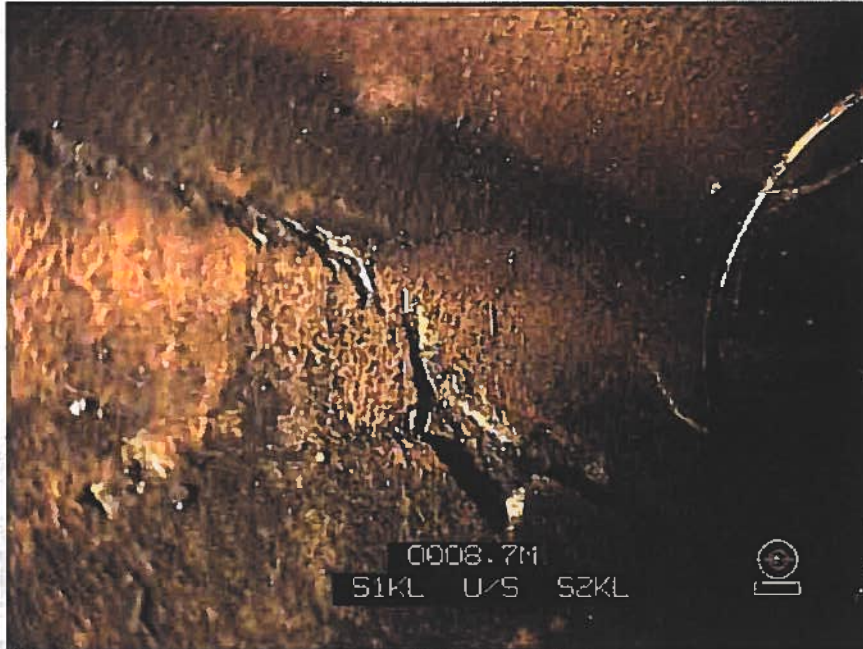
1, 00:02:11, 8.70 m Fracture, circumferential from 7 o'clock to 10 o'clock
