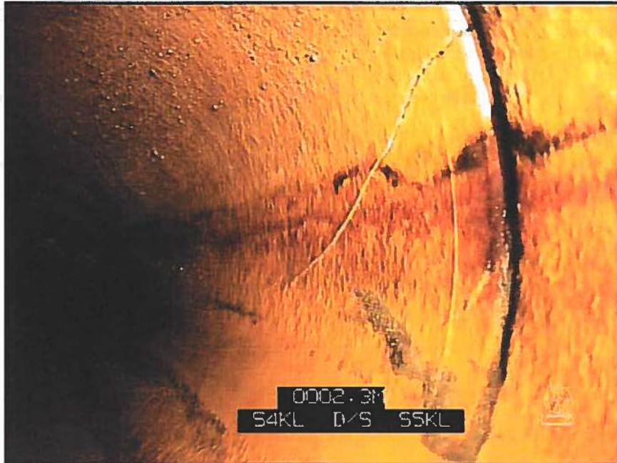
1, 00:00:49, 2.30 m Fracture, circumferential at joint from 5 o'clock to 6 o'clock
