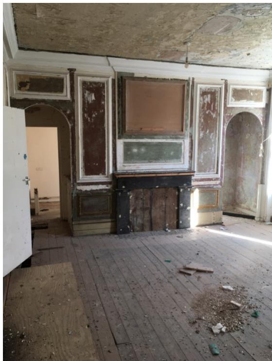
7 FIRST FLOOR PANELLED ROOM (to be repaired)
