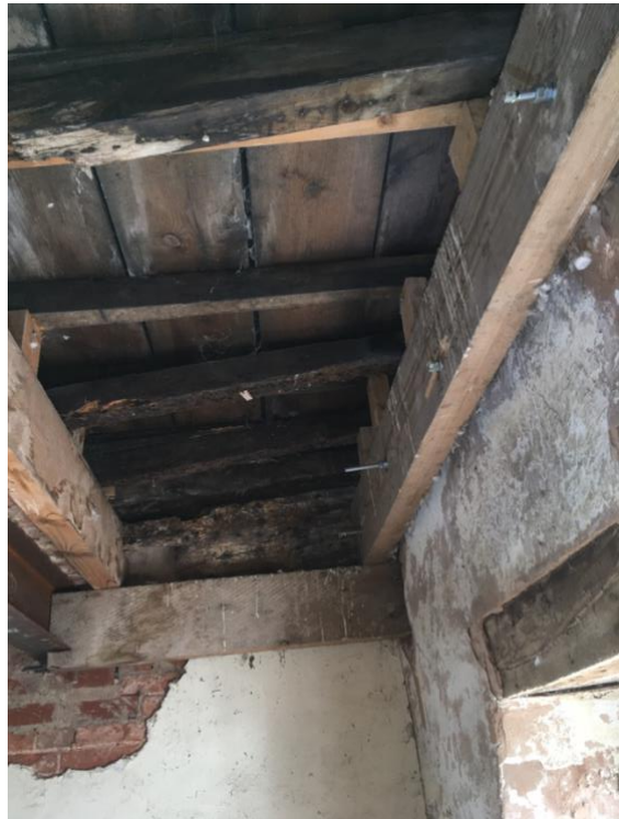
6 UNDERSIDE OF GUTTER (to be replaced)
