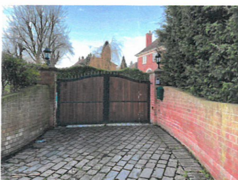
Photograph 9 - Taken Outside the Double Gates. The Gates shown has been decorated due to poor conditions and timber infill panelling added for security.
