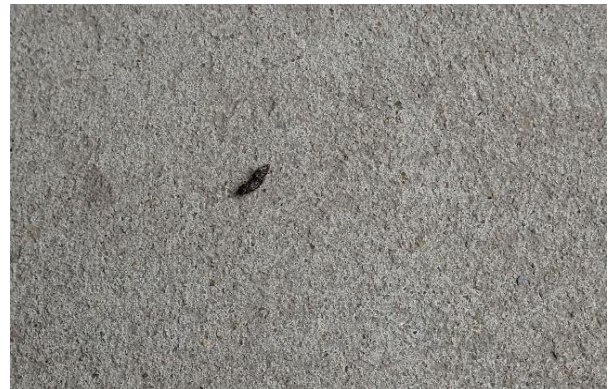
Pipistrellus type dropping on floor of building
